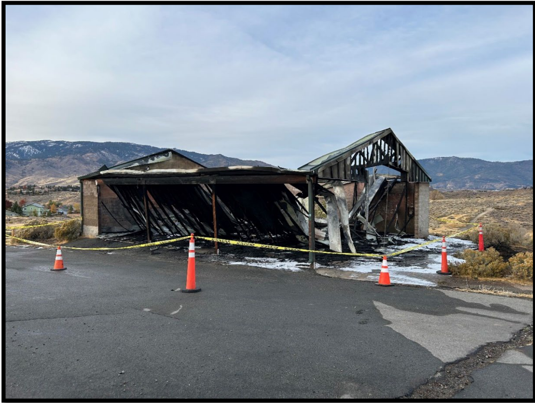
Exhibit A. Pictures of the damaged shade structure
