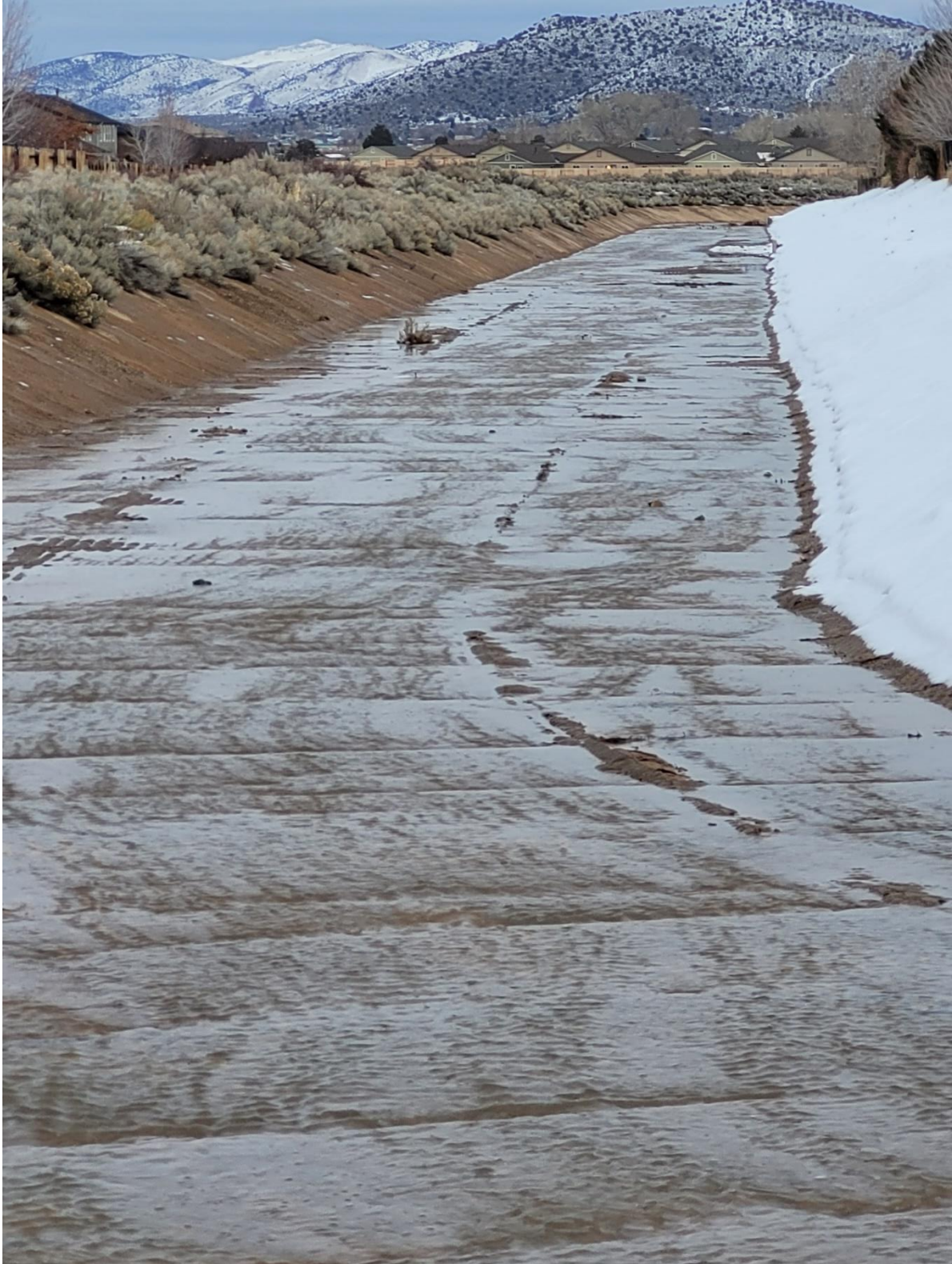
Inspection Site 10) Downstream channel running toward Swan Lake. It is clean with no obstructions to impede water. (1/11/2023)
