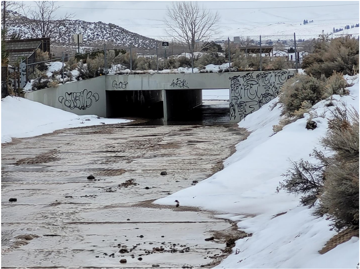
Inspection Site 9) Drainage ditch north of Tulear St. This is the road crossing under Military Rd. It is clear of debris and flowing without obstruction. (1/11/2023)
