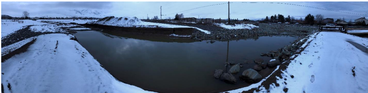
Inspection Site 8) Channel leading into the road crossing at Military Rd. is clean with no obstructions to impede water. It is clear of debris and functioning as designed. (1/11/2023)
