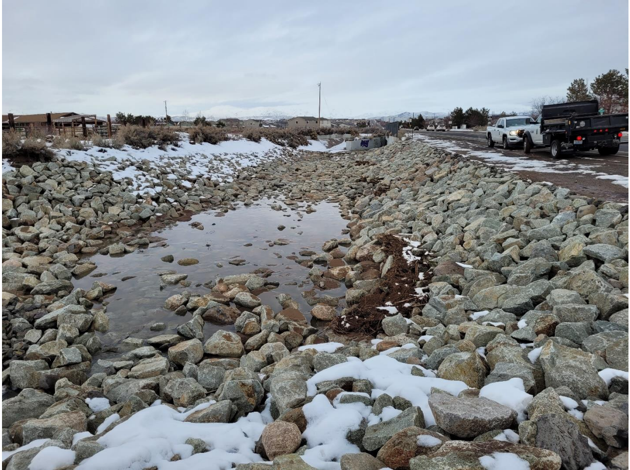
Inspection Site 7) Completed channel downstream of the construction site heading toward Military Rd. It is clean with no obstructions to impede water. (1/11/2023)
