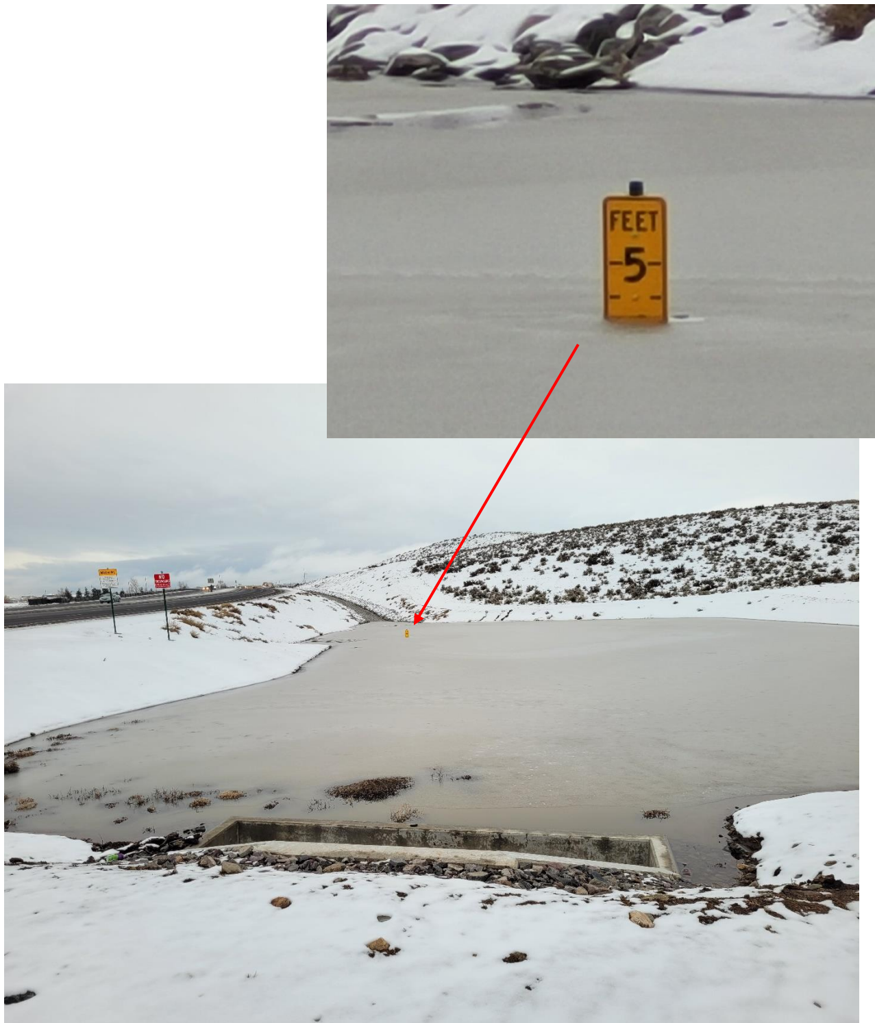
Inspection Site 1) Retention structure south of 8075 Lemmon Dr. The water level inside the basin is below the designed outlet structure and is in no danger of overtopping. (1/11/2023)
