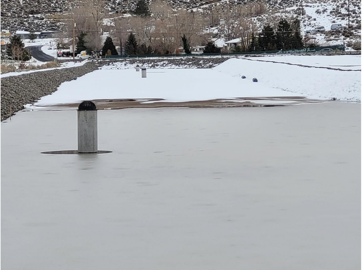
Inspection Location 6) Construction site south of 8730 Military Rd. This retention area is still under construction and no danger of overtopping. (1/11/2023)
