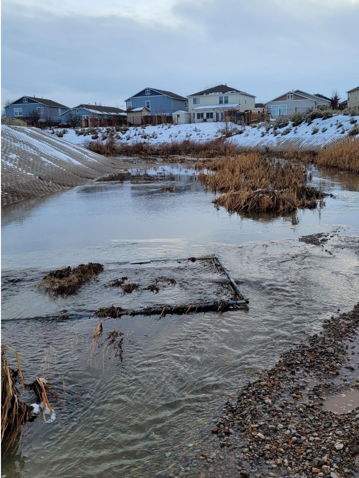
Inspection Site 5) Picture at the confluence of Lemmon and Military Rd. drainage channels, looking towards Lemmon Valley Road. Some debris present however the channel is functioning as designed and is not in danger of overtopping. (1/11/2023)
