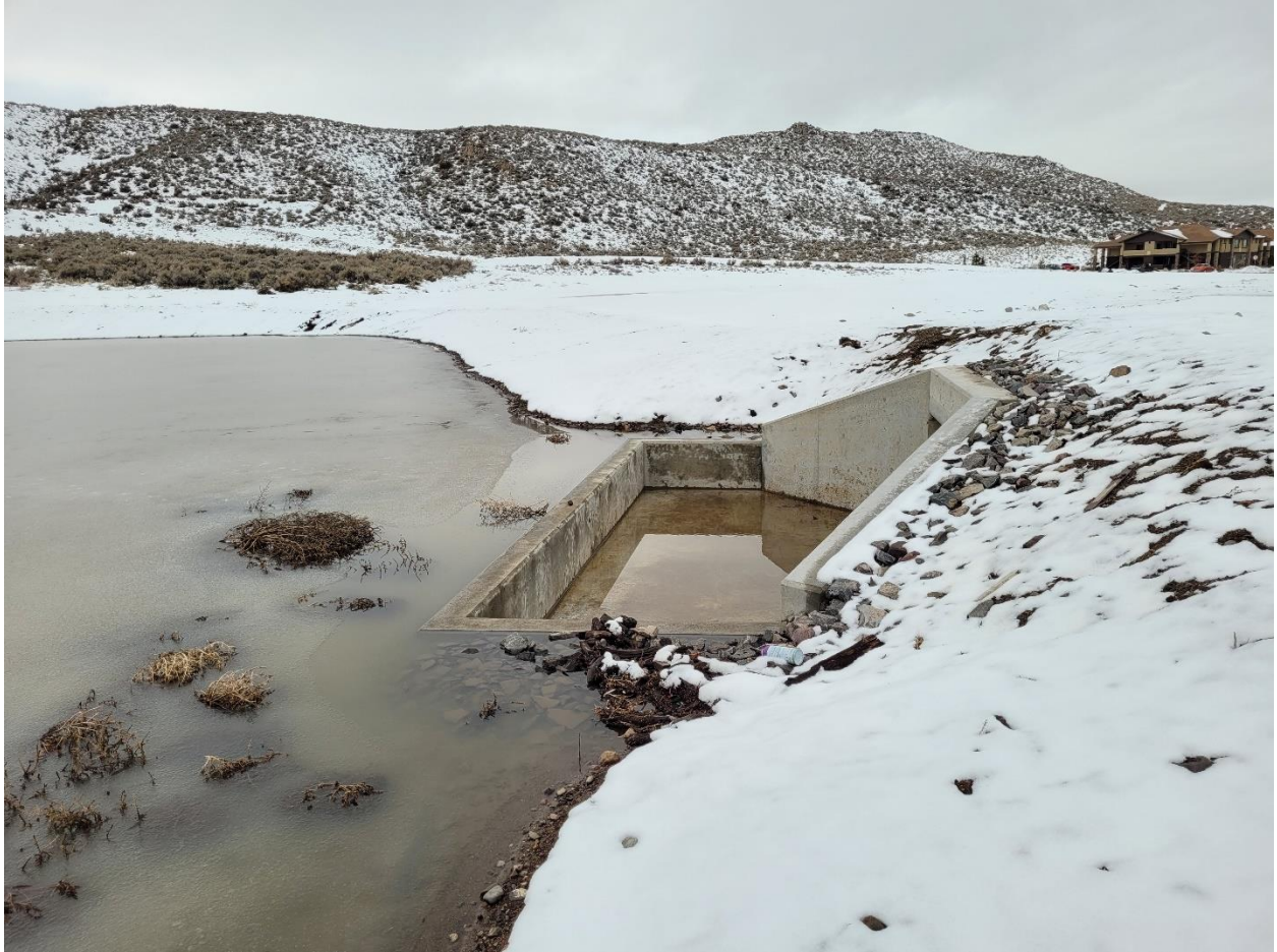
Inspection Site 1) Picture of the outlet structure. It is clean with no obstructions to impede water. (1/11/2023)
