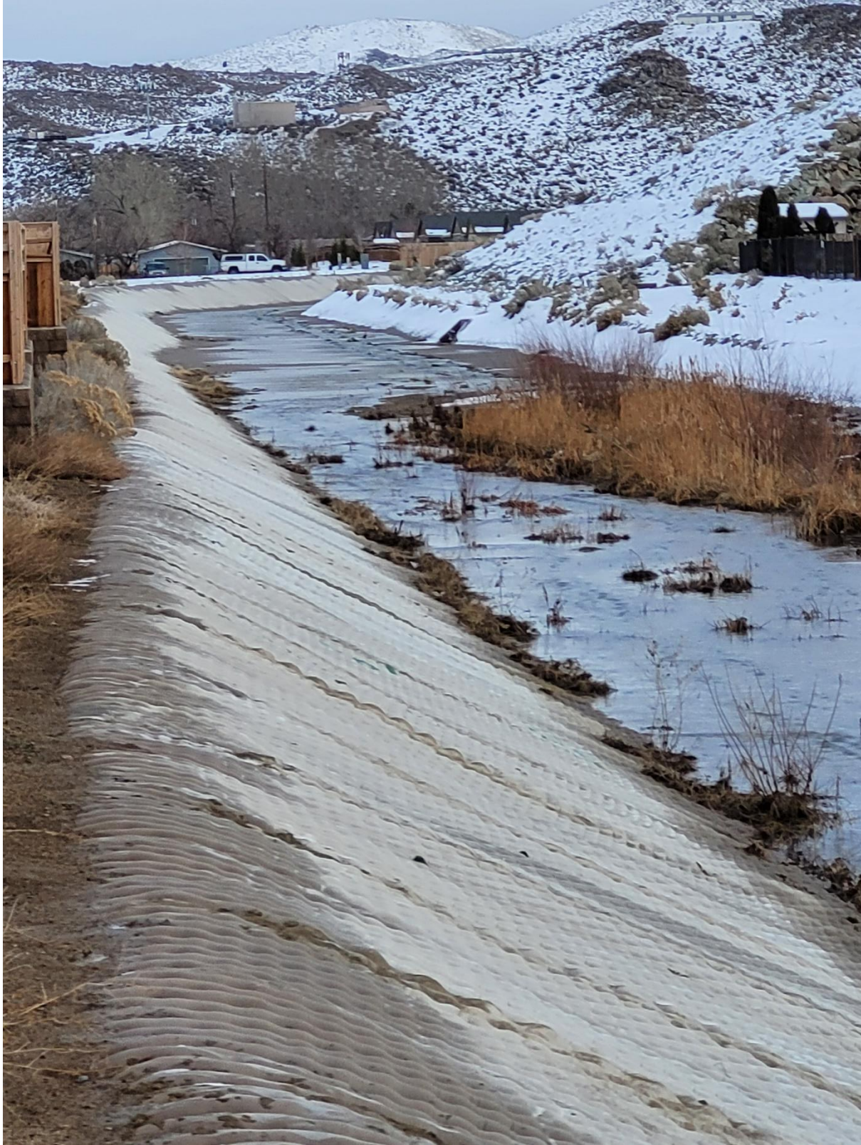
Inspection Site 4) Downstream of Lemmon Dr. road crossing. The channel is in no danger and functioning as designed. (1/11/2023)
