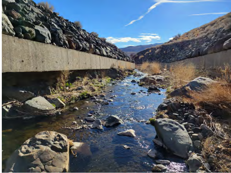
Photo 3. Galena Creek looking downstream in the section of engineered channel under the I-580 bridge. Galena Creek is actively migrating laterally within the section of engineered channel and eroding under the concrete walls on both banks.
