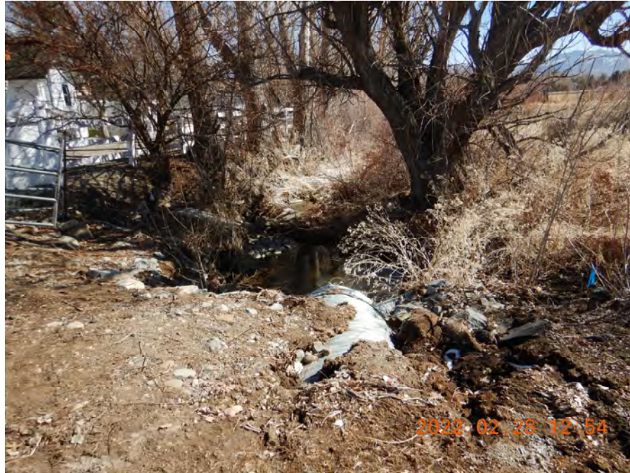
Photo 5. Soil eroding from the downstream end of the 48-inch corrugated metal pipe culvert at the end of Bonde Lane and entrance to Anderson Regional Park.
