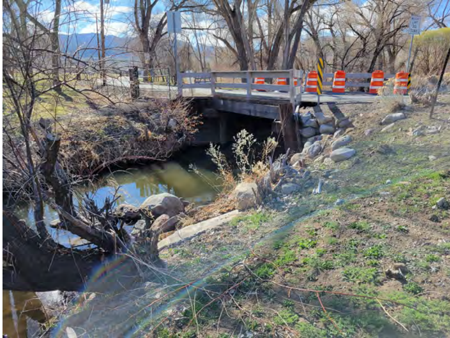
Photo 1. Rhodes Road crossing. There is active erosion near the footing of the wooden structure. Washoe County is currently working through the design phase to replace the existing structure.
