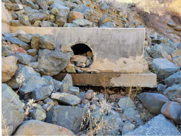
Photo 1. An upstream storm drain outfall is blocked with debris and rocks. The outfall footing is being undermined.
