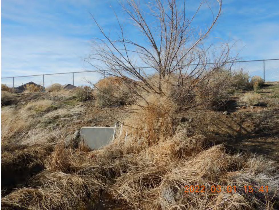
Photo 5. Overgrown storm drain outfall near Miguel Sepulveda Elementary School.
