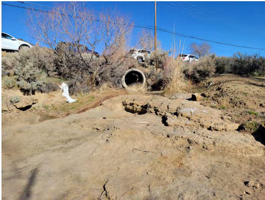
Photo 4. Existing 48-inch culvert outfall from Steamboat Ditch discharges to a bare unconfined area to the west of Steamboat Creek.
