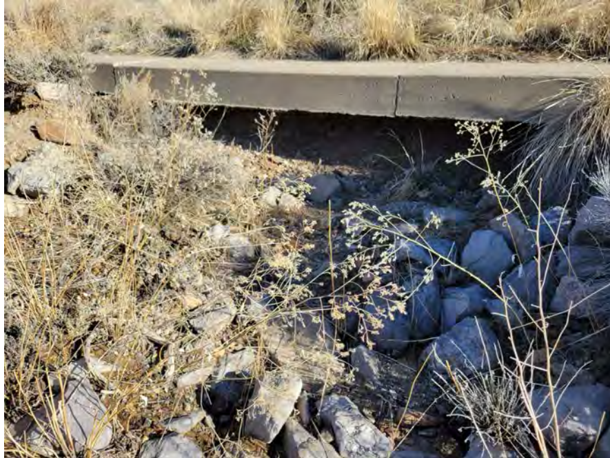
Photo 1. Standing downstream and looking upstream at concrete grade control structure. The historic channel crossed the existing structure at this location until the formation of western channel (Photo 2). Flow from Chalk Creek has undercut the existing concrete.
