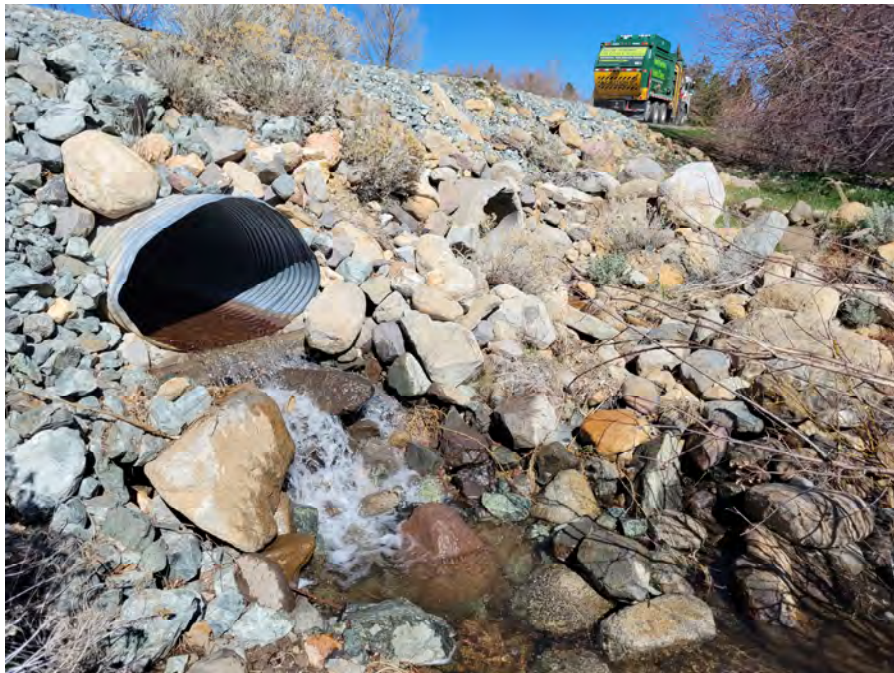
Photo 2. A 38-inch by 54-inch arch corrugated metal pipe (CMP) and 36-inch concrete culvert convey flow under Callahan Ranch Road. The CMP culvert inverts are set below the concrete culvert and convey low flows.
