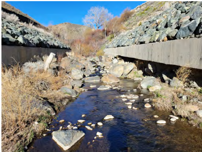
Photo 2. Galena Creek looking upstream in the section of engineered channel under the I-580 bridge. The concrete walls are undermined and stand 4 feet tall. It was estimated that the northern wall (right) has been undermined between 4 and 8 feet from the front face and is suspended up to 6 feet above the existing channel bottom. Access along the way was limited, and observations were made from the southern bank.
