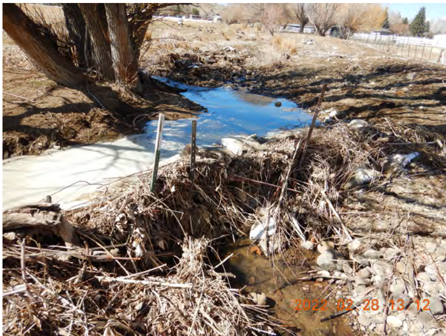
Photo 4. Channel bifurcates at this location. Concrete ready-mix bags and t-post have been used to block flow towards the northeast and limit flow entering the private parcel to the north. Debris has collected on the makeshift improvised diversion structure.
