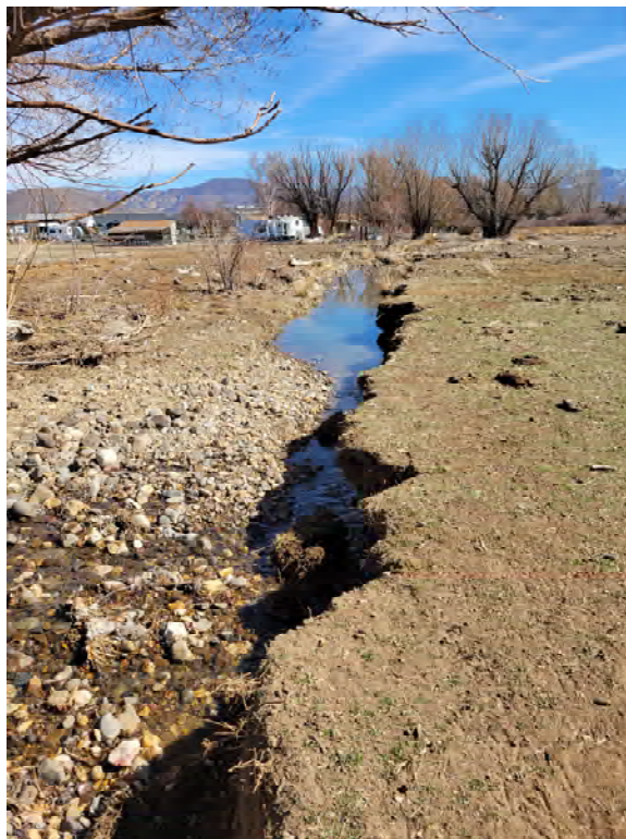
Photo 2. Looking east standing at the top of the southern bank. The southern bank is actively being eroded and soil is slumping into South Evans Creek.
