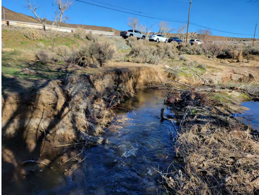
Photo 3. Steamboat Creek looking downstream, immediately downstream of the existing weir structure. The channel is actively eroding the left bank. The bank is up to 5-feet tall in this location. The banks in this area were previously documented to be 3-feet tall.
