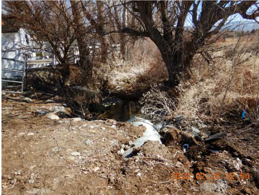
Photo 5. Soil eroding from the downstream end of the 48-inch corrugated metal pipe culvert at the end of Bonde Lane and entrance to Anderson Regional Park.
