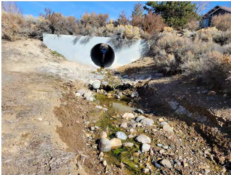
Photo 4. Valley Wood Drive culvert with 18-inch headcut downstream of the grouted riprap apron.
