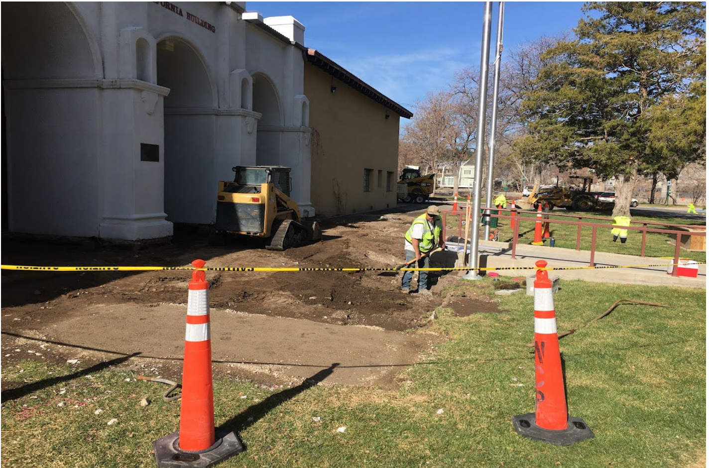
About Picture: Replacement of ramp at California building to become ADA compliant
