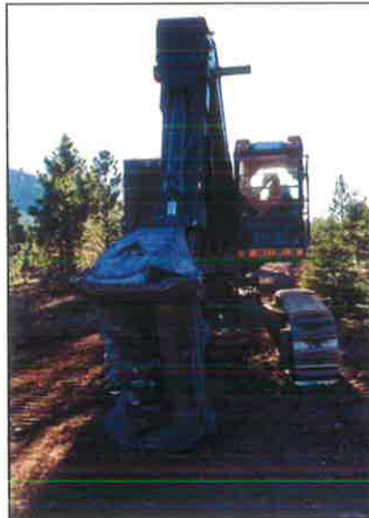
Figure 6.1 – Boom mounted masticator. Allows operator to grind up brush with pin point accuracy, while minimizing the environmental impact.
