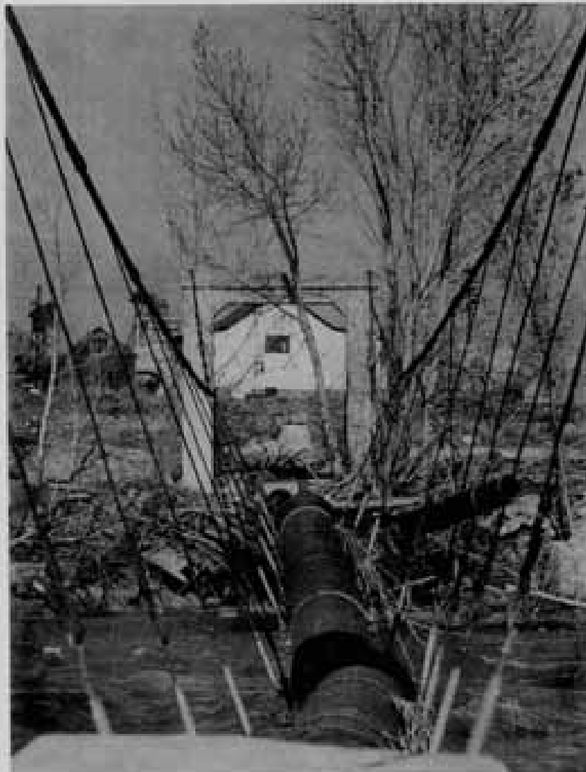
Figure 26. Flood-carried debris seriously damaged the main sewerage pipeline bridge east of Wells Avenue, November 1950 (Gene Christensen Photo*)
