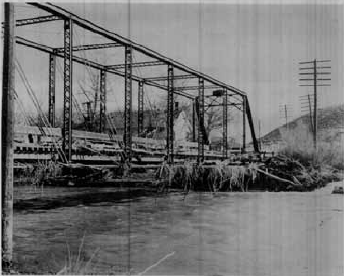
Figure 25. Debris on Mayberry Drive Bridge after the December 1955 flood. (Photo courtesy of the Washoe County Engineer's Office)
