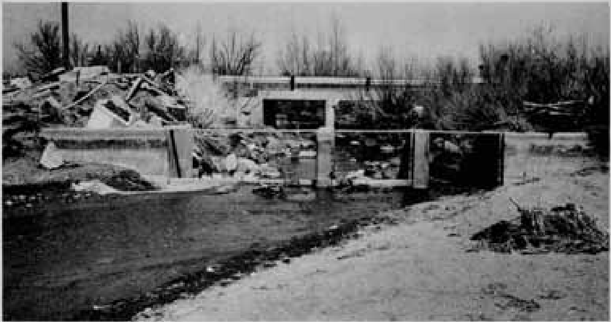
Figure 28. Obstructive irrigation structure on Dry Creek. Bridge at East Peckham Lane in background.
