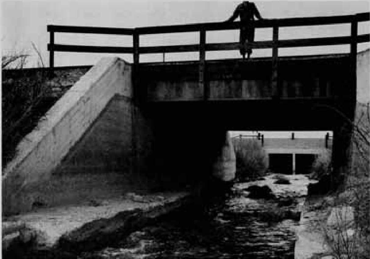
Figure 32. Southern Pacific railroad bridge crossing of North Truckee Drain. Box culvert at Interstate 80 in background.
