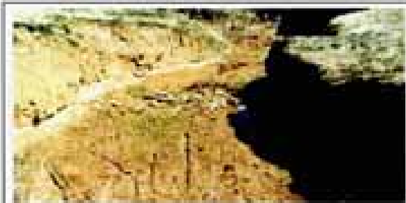
Degraded drainageway as a result of upstream development Courtesy Urban Drainage and Flood Control District, Denver
