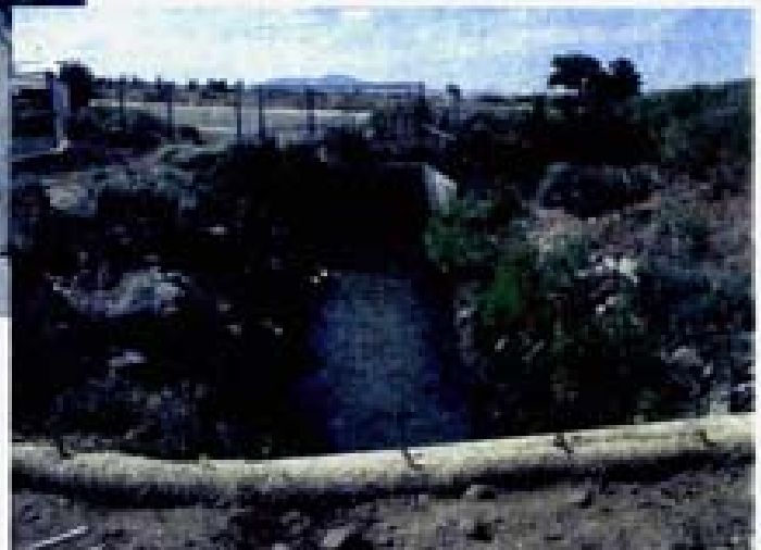
Figure 6. Looking north at the Steamboat Ditch. The road in the background is Arrow Creek Parkway, and the culverts shown in Figures 4 and 5 above flow from right to left under this.
