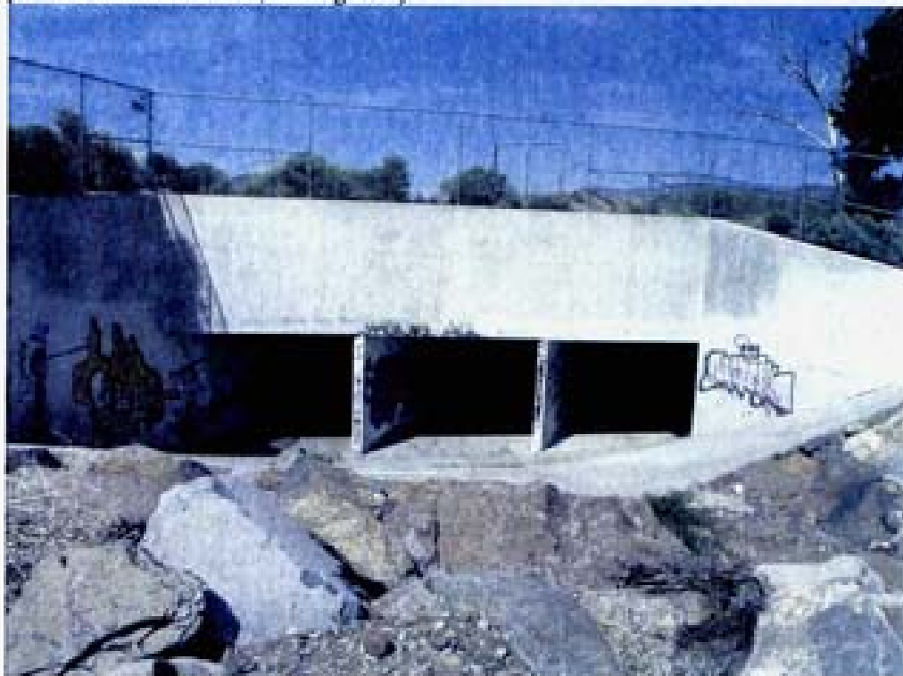
Figure 4. Looking northeast (downstream) at the box culverts under Arrow Creek Parkway. The approach is steep because these culverts also cross under Steamboat Ditch (flowing from left to right past the chain link fence, see Figure 6).
