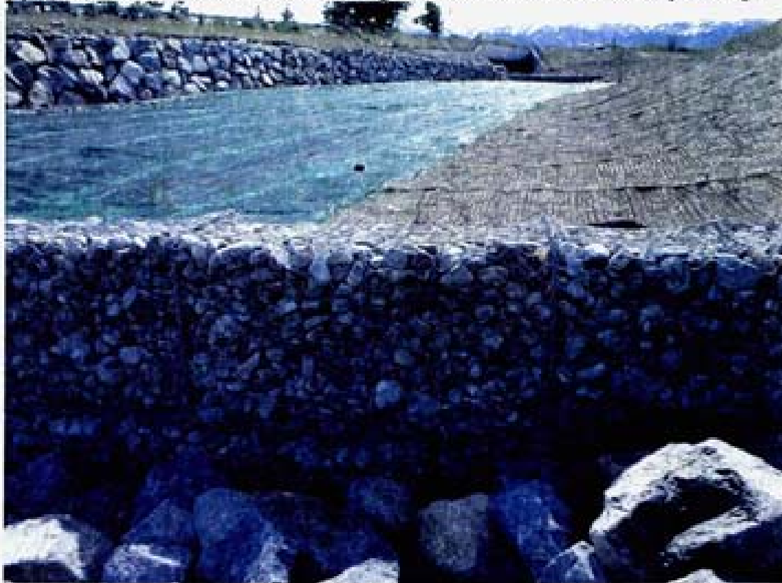
Figure 3. Detail showing a typical gabion drop structure and geotextile lining, looking east (upstream). The three box culverts in the background are the Arrow Creek Parkway crossing.
