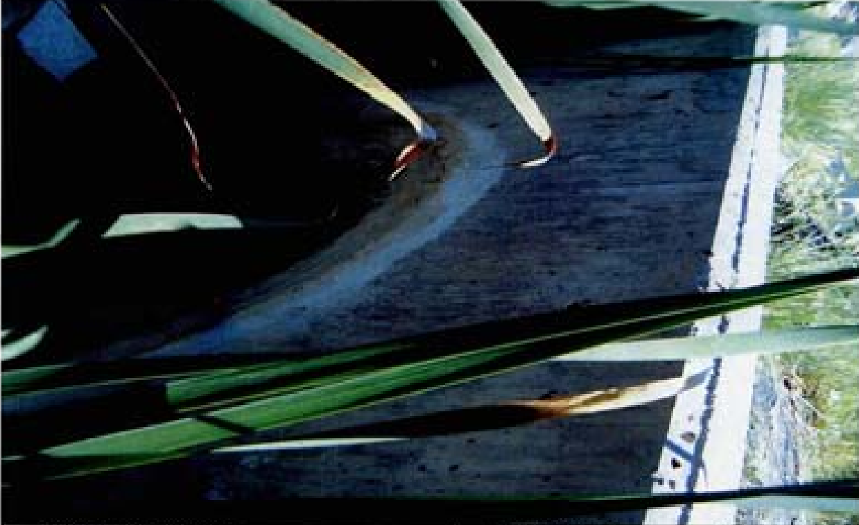
Title: Site 13 - SD out of Village 16 File: HPIM2274.JPG Date: 8/22/2006 12:45 Desc: Slide: 2272 Facing Easterly, outlet of RCP and headwall. The RCP/headwall interface has been refinished. Air voids are visible from inadequate vibration during forming. Form rod spacers have not been removed. Some repatching of headwall is visible in top left of photo.
