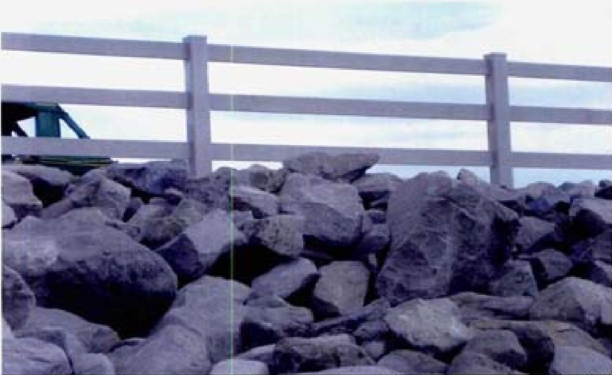
Title: Site 6 - Channel C-7 File: P1010175.JPG Date: 9/18/2006 15:17 Desc: Slide: 1010175 Facing Southerly; outlet of PVC culverts from Photo 1010174.
