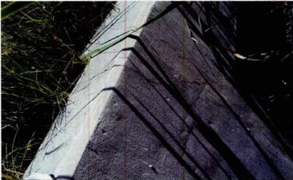
Title: Site 18 - RCB outlet across from Damonte High School File: HPM2287.JPG Date: 8/22/2008 13:34 Desc: Slide: 2285 Facing SEasterly; intersection of headwall/wingwall. This is a crack that runs from top to bottom and appears to run from front to back of the wingwall.
