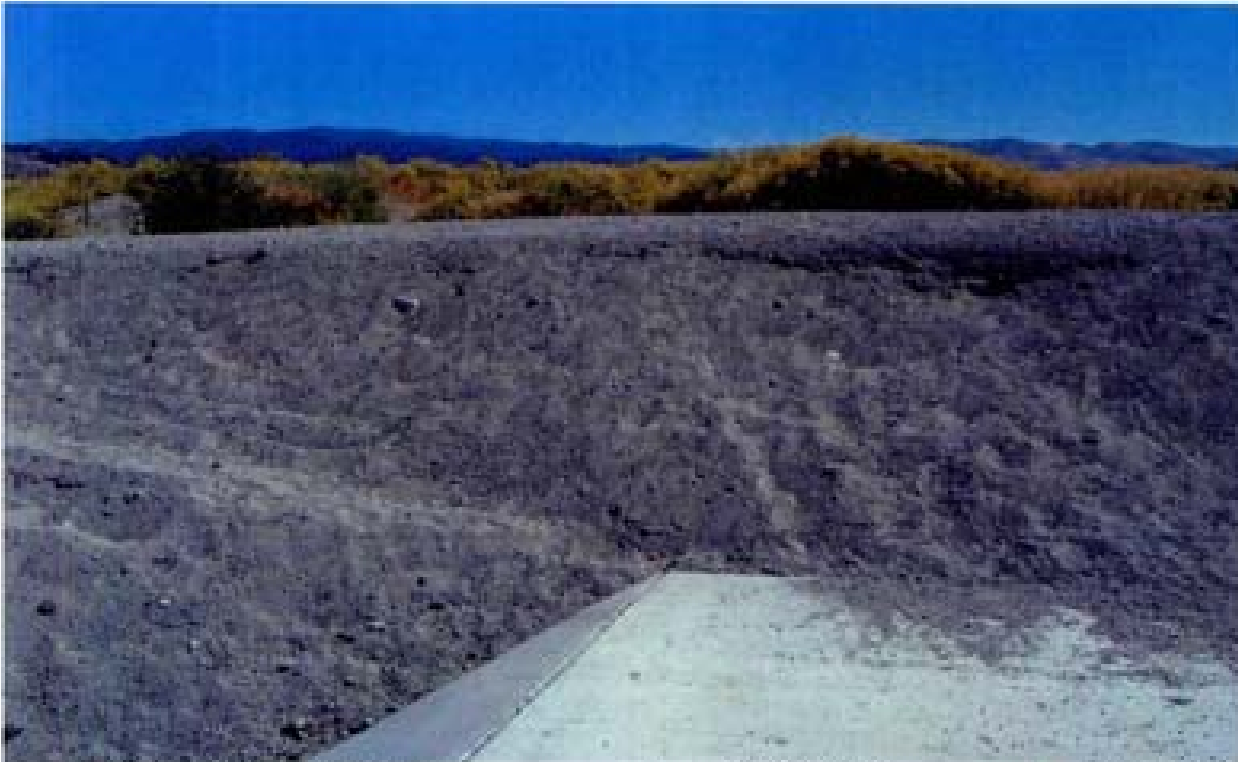
Title: Site 1 - Detention basin diversion structure File: HP0M2191.JPG Date: 8/15/2006 15:26 Desc: Facing Southerly; same location as Photo 2191 at south end of diversion structure. Note where non-cohesive sand erosion has exposed the cohesive layer of soil cement in upper right center of photo.
