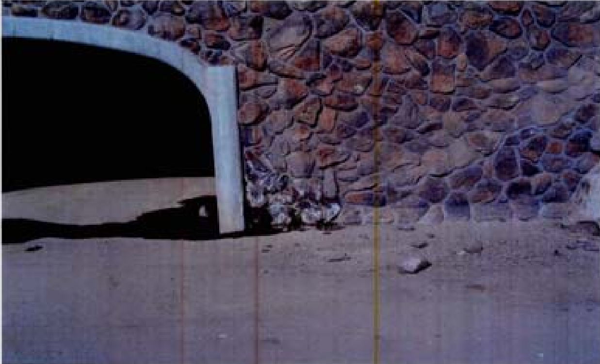
Title: Site 3 - Detention basin outlet structure File: HPM2242.JPG Date: 8/22/2006 9:26 Desc: Slide: 2242 Facing Westwely; water seepage from behind wall. This water appears to be associated with the irrigation of the greenspace on the bridge.
