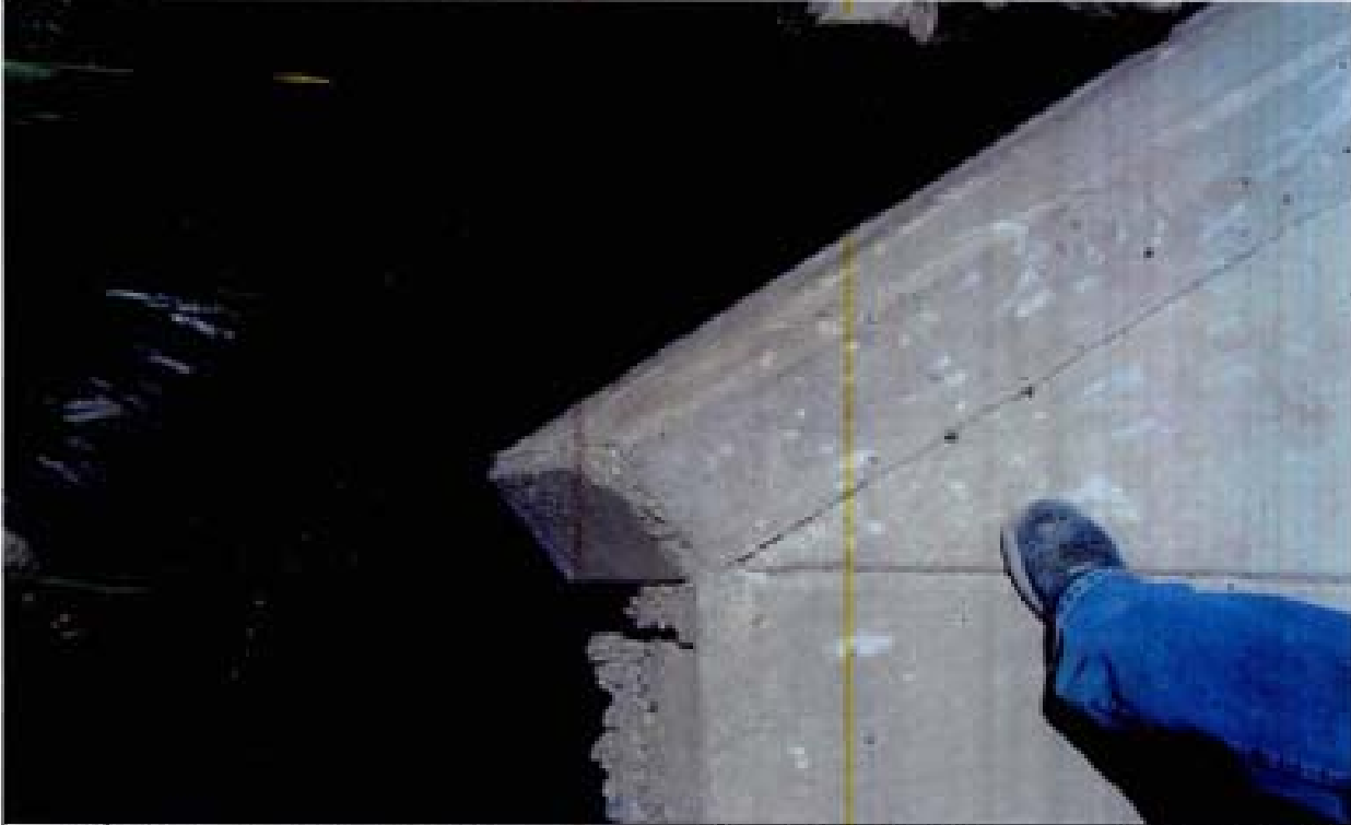
Title: Site 1 - Detention basin diversion structure File: HPM2194.JPG Date: 8/15/2006 15:30 Desc: Slide: 2194 looking down at interface of flared wing wall and sloping PCC apron of diversion structure. No cut off wall constructed.
