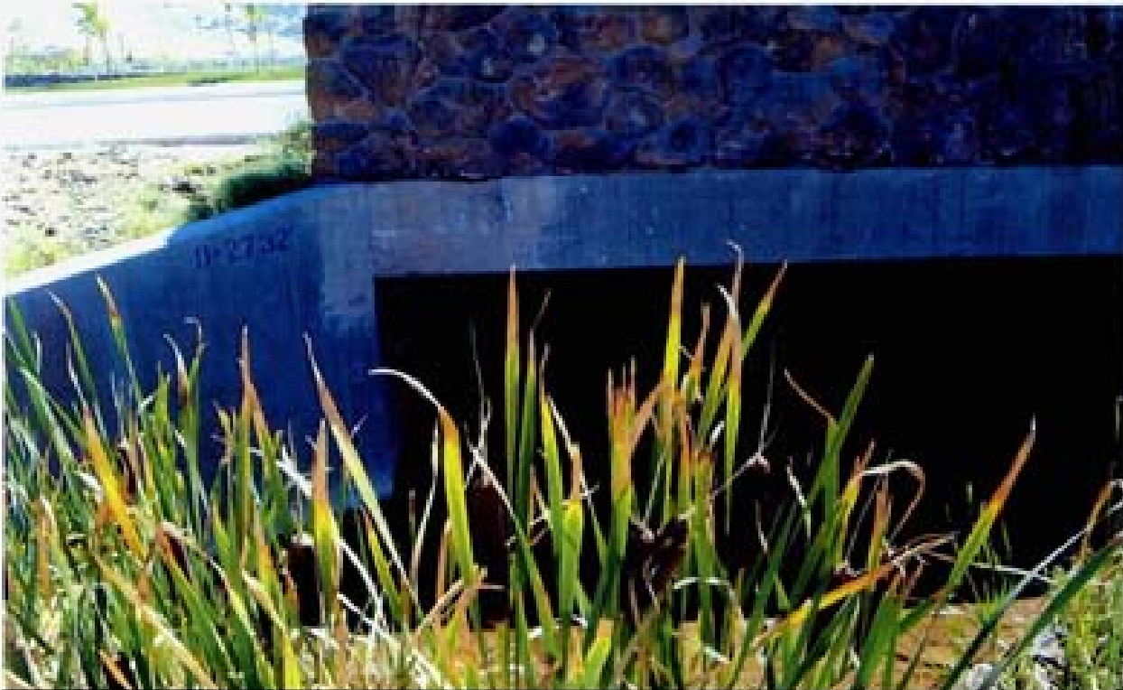
Title: Site 19 - Intersection of Rio Wrangler and Steamboat Parkway File: HPIM2294.JPG Date: 8/22/2006 13:49 Desc: Slide: 2291 Facing Southerly, outlet of five RCB's under Steamboat Parkway. The designation B-2732 is an NDOT numbering indication that this bridge has been inspected by NDOT and added to the national Register of Bridges.
