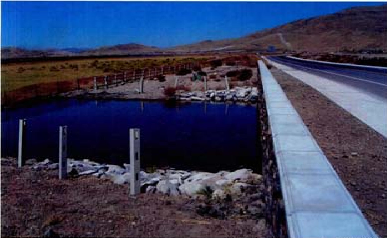
Title: Site 20 - bridge crossing under the Winder South of Steamboat Parkway File: HP1M2298.JPG Date: 8/22/2008 14:01 Desc: Facing Northerly; outlet of 4 RCB's. Riprap stabilization at outlet. Riprap is angular with fractured faces and good length/width ratios of ~ 2:1. There is no visible signs of bedding or geotextile underlayment. End of channel has a fiber roll installed that is causing the backwater and appears to have been installed as an sediment control BMP. The riprap extends about ~12 feet down from the outlet.
