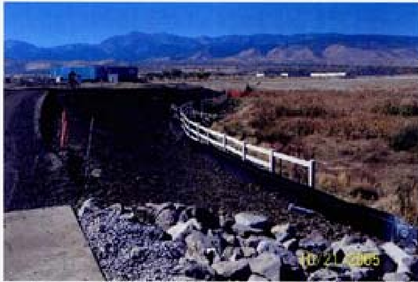
Photo 87, 10/21/05 - Silt fence protecting upper southern end of wetland 015. View looking west with a portion of the drop structure for channel C-7 in the foreground.
