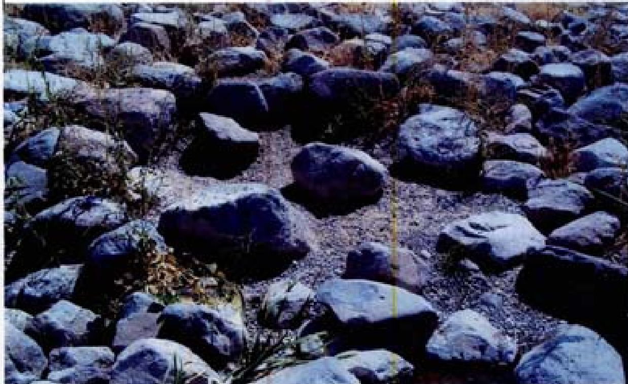
Title: Site 15 - weir from DE3 to DE1 pond File: HPM2306.JPG Date: 8/23/2008 14:15 Desc: Slide: 2302 Facing SEasterly; southern side slope of overflow weir. The rock has been displaced exposing the gravel bedding underlayment. Rock in this section appears to be only one layer thick with the apparent median rock size ~12 inches. Same comments as Photo 2308 apply.
