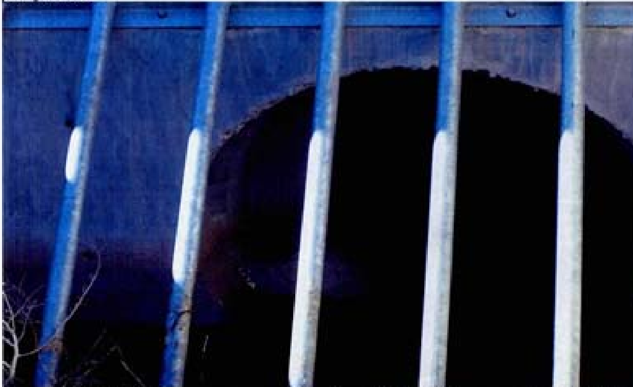
Title Site 9 - Channel C5-B File HP1M2224.JPG Date: 8/15/2006 16:45 Desc: Facing Northerly; close up of RCP inlet on right. Note the bell end of the pipe was formed in the headwall with about a 15 degree skew. The right side of the pipe is flush with the front face of the headwall and the left side of the pipe is approximately flush with the back of the headwall...6' from the front face. Note PCC "blowout" in lower left of pipe impedes on flow area of pipe inlet.
