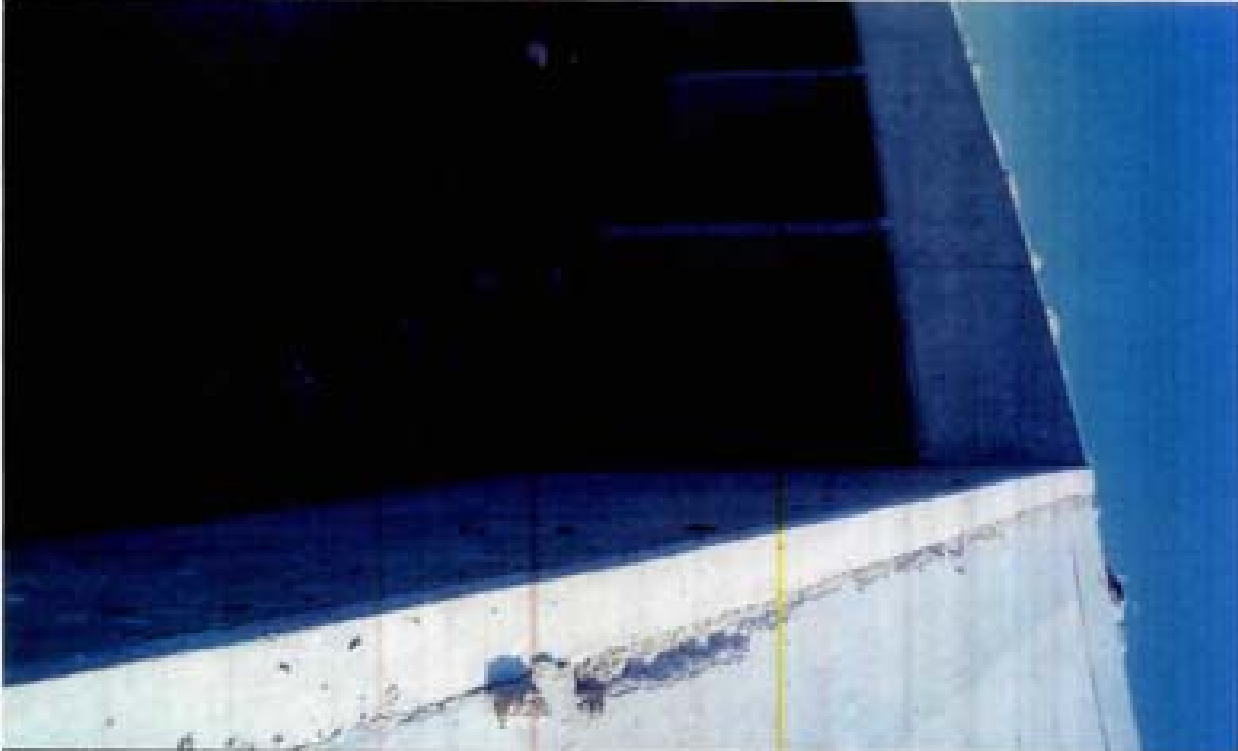
Title: Site 1 - Diversion Structure File: HPM2234.JPG Date: 8/22/2008 8:45 Desc: Facing Northerly; interface of sloping PCC apron of diversion structure and flared wingwall. Note degradation of PCC apron.
