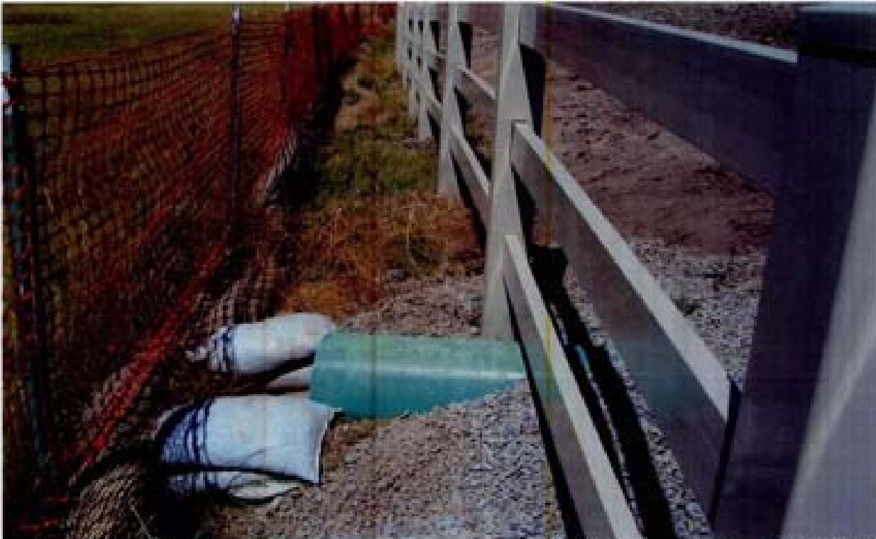
Title: Site 21 - PVC SD outlet File: HP1M2301.JPG Date: 8/23/2006 14:03 Desc: Slide: 2297 Facing Northerly; outlet of PCV SD (?). Outlet of PVC pipe. Source of pipe not apparent in field walk.
