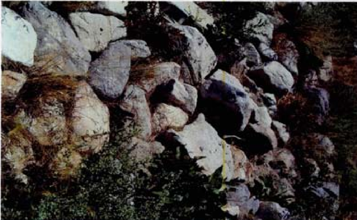
Title: Site 3 - Detention Basin File: HPM2201.JPG Date: 8/15/2006 15:50 Desc: Same location as Photo 2200; rip rap at inlet to headwall/RCP detention low flow outlet. Steel construction stake in center of rip rap is potential tripping hazard.
