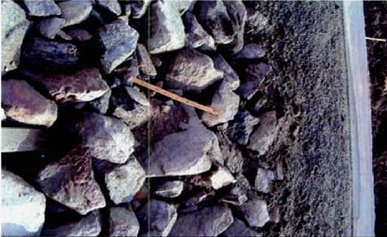
Title: Site 7 Channel C-5 File: HPIM2587.JPG Date: 11/12/2006 11:03 Desc: Facing Easterly, riprap at end of first grade control sill. Some hydroseed on the bank.
