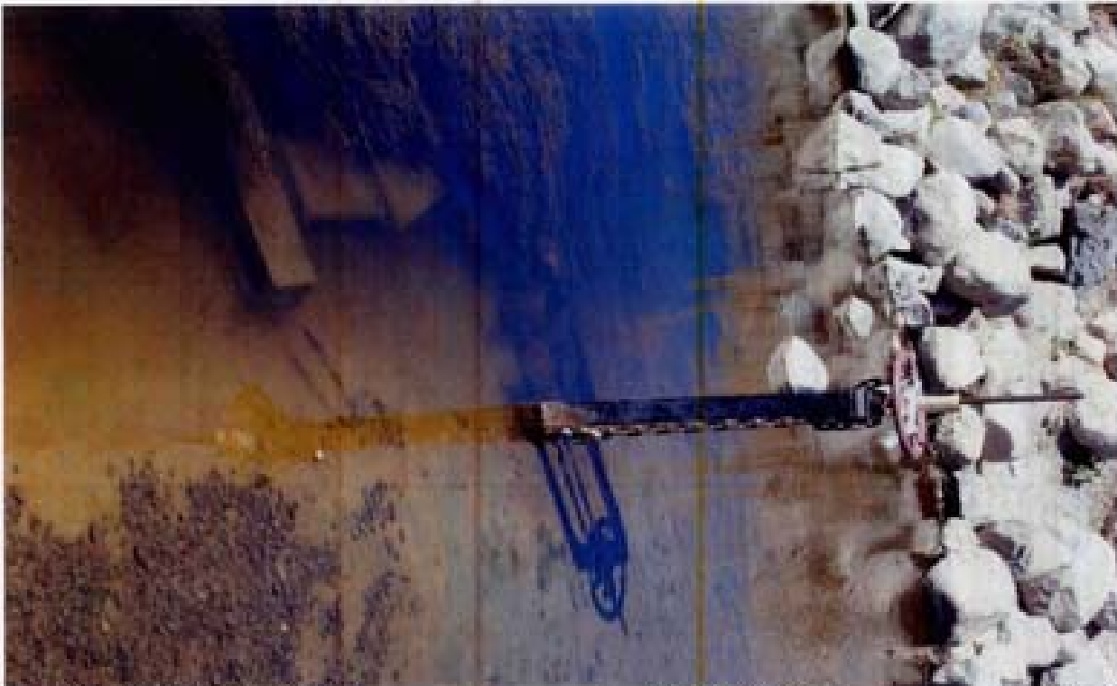
Title: Site 15 - weir from DE3 to DE1 pond File: HPM2305.JPG Date: 8/23/2008 14:14 Desc: Slide: 2301 Facing NWesterly; low flow gate valve in PCC weir. The valve handle lock/chain appears to be broken. The low flow inlet is blocked with rock. Masonry blocks/tetons in upper left of photo.
