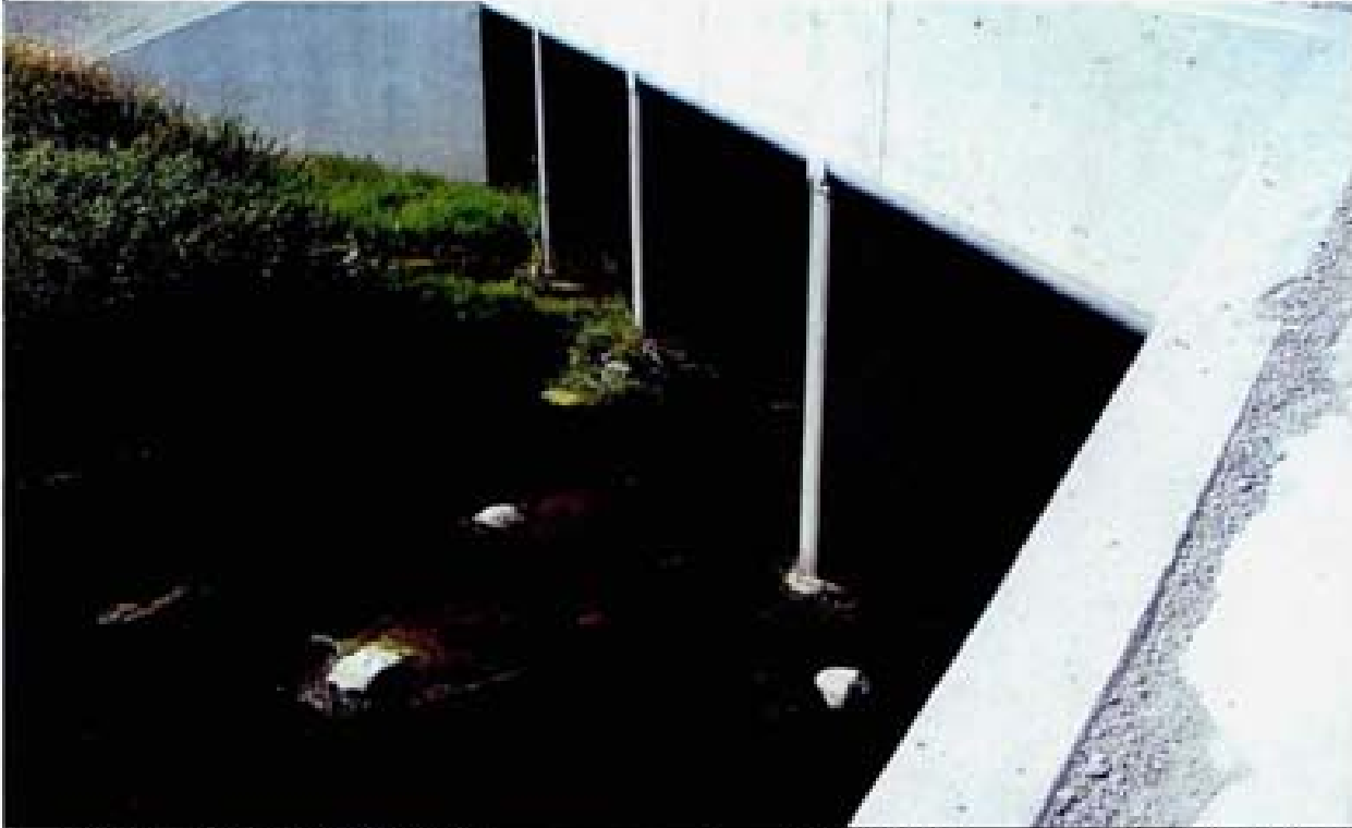
Title: Site 1 - Detention basin diversion structure File: HPM02196.JPG Date: 8/15/2008 15:33 Desc: Slide: 2196 Facing Westerly; inlet to RCB culverts. Note spalled concrete of sloping PCC apron in left foreground.
