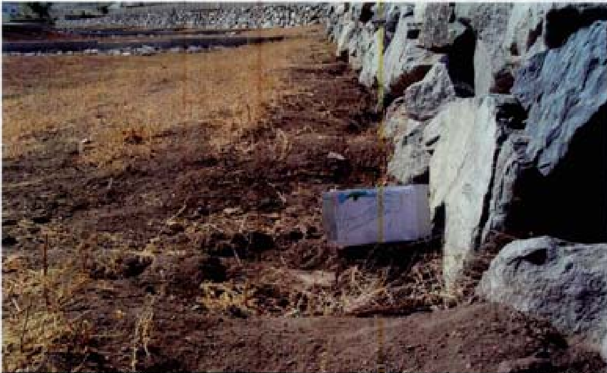
Title: Site 11 - Channel SE-8A File: HPM0250.JPG Date: 8/22/2006 10:09 Desc: Slide: 2249 Facing SEasterly; exposed end of grade control sill along south side of channel. Note that the PCC control sill ends -1.5 feet from the bottom of the rocky wall.
