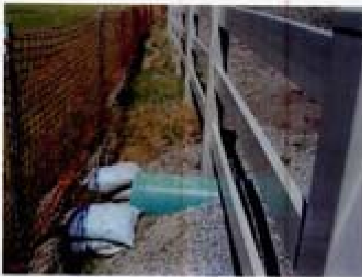
PVC storm drain outlet
