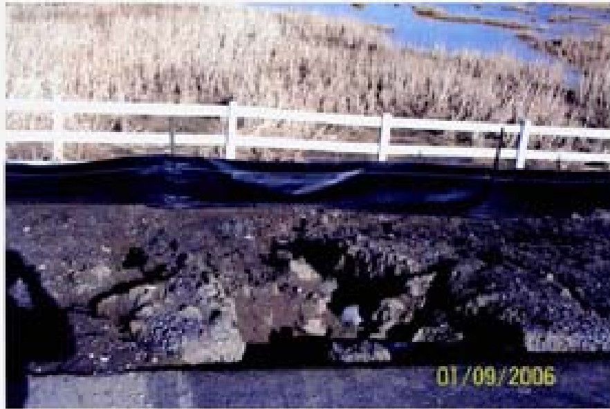
Photo 08, 1/9/06 - The erosion shown in this photo is the result of an impermeable surface (the bike path) located directly above a steep fill slope. A gravel or sand buffer at the edge of the pavement would help to disperse the runoff and the slope should be a maximum 3H:1V. The unprotected slope should also be stabilized as soon as possible with mulch or another similar BMP.
