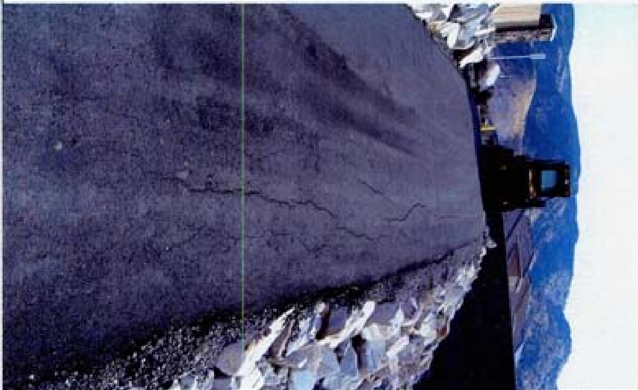
Title: Site 10 W-3 Channel File: HPM2591.JPG Date: 11/12/2008 11:11 Desc: Slide: 2591 Facing Southerly: access ramp into beginning of W-3 channel. AC is cracking.
