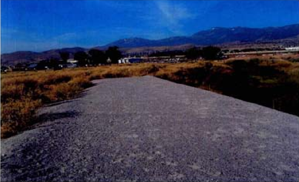
Title: Site 1 - Diversion Structure File: HPIM2240.JPG Date: 8/22/2008 8:55 Desc: Facing Southerly; South end of the soil cement where it meets the natural grade on upstream, eastern bank of Steamboat Creek. Note coarse sandy, non-cohesive material.
