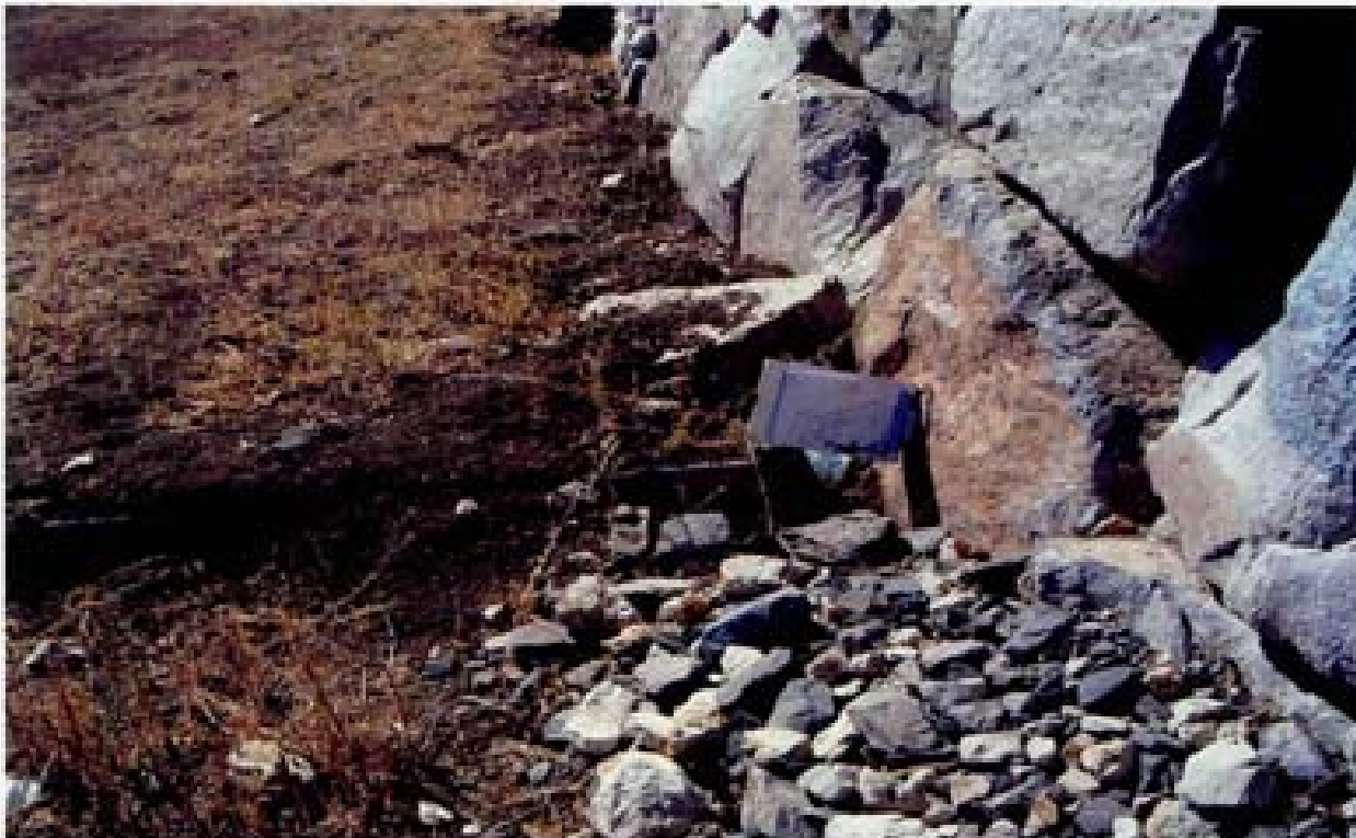
Title Site 11 - Channel SE-8A File HPIM0252.JPG Date 8/23/2008 10:11 Desc Slide 2251 Facing SEasterly, exposed end of grade control sill along south side of channel. Note that the PCC control sill ends ~1 feet from the bottom of the rocky wall. No riprap protection.
