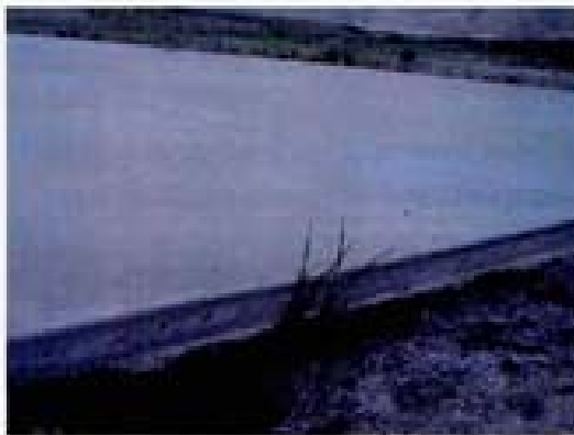
Undercutting of PCC apron
