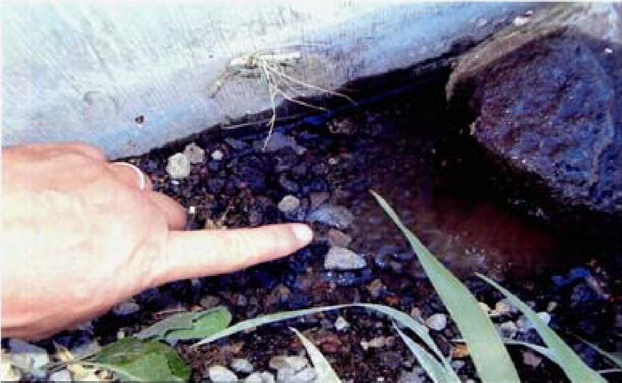
Title Site 4 - DE5 Wetland File HPM2207.JPG Date 8/15/2006 16:01 Desc: Facing Westerly; same as Photo 2206. Close up of water seeping out from beneath headwall.
