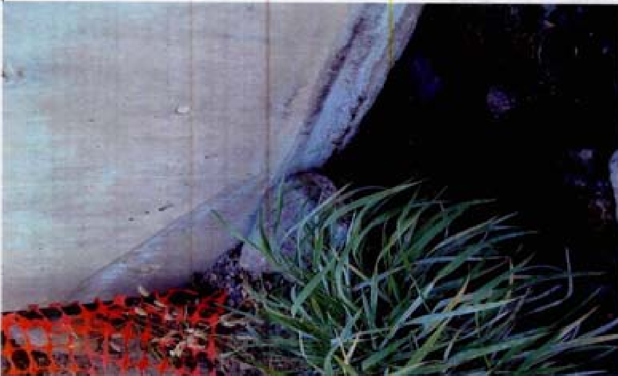
Title Site 4 - DES Wetland File HPM2206.JPG Date 8/15/2008 16:00 Desc: Facing Westerly; left corner of headwall shown in Photo 2205. Water is seeping out of the ground under the headwall... beneath rock in center of photo. See Photo 2207.
