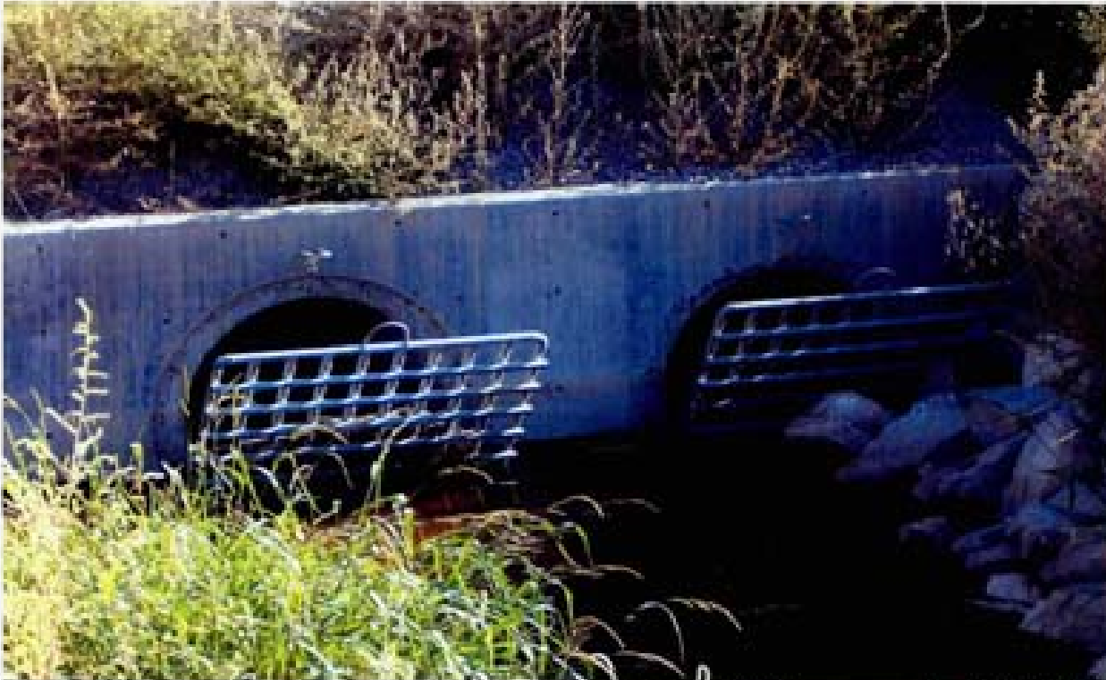
Title: Site 9 - Channel W1-B File: HPM2227.JPG Date: 6/15/2006 16:53 Desc: Facing southerly; Downstream end of twin 36 inch RCP's under Rio Wrangler. Poorly constructed RCP/headwall interface. PCC has flaked away from RCP pipe on left. Form rod holes not filled. Safety grates no longer applicable to current Reno Standard Details. Slide: 2227
