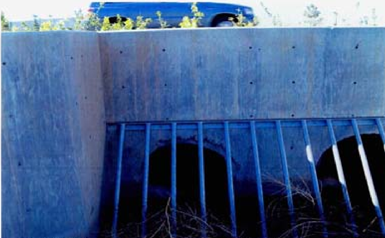
Title Site 9 - Channel C5-B File HP1M2223.JPG Date: 8/15/2006 16:42 Desc: Facing Northerly; inlet of twin RCP's. This headwall has been very poorly formed and has PCC flaking away from the RCP/headwall interface from both pipes. Large slumps of PCC blew out from the form and are obstructions to the entrance to the pipes as can be seen in the lower left of each pipe. There are no nuts on the bolts securing the trash rack.
