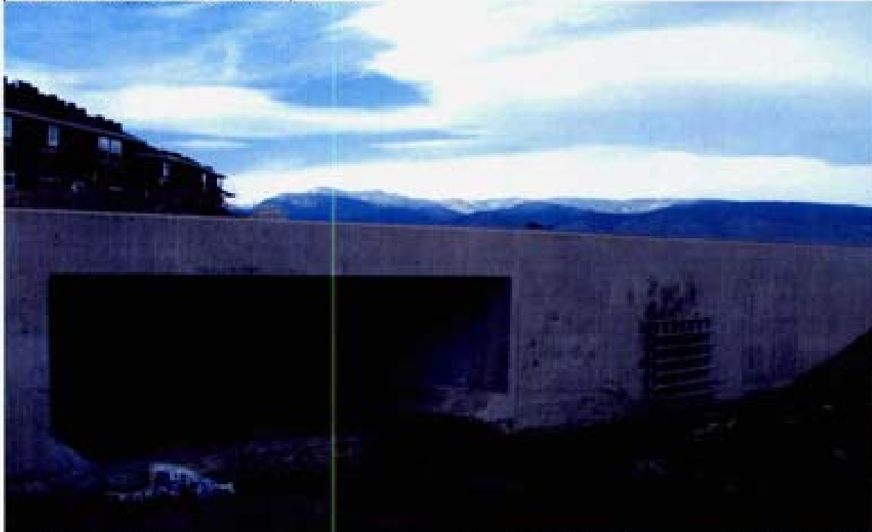
Title Site 7 - C-5 Channel File P1010156.JPG Date 9/18/2006 15:17 Desc Slide 1010156 Facing SWesterly; outlet of RCB into c-5 channel. Same location as Photo 1010155. Safety grate on RCP on SD outlet from headwall. There is no riprap outlet velocity protection at the outlet of the RCB.
