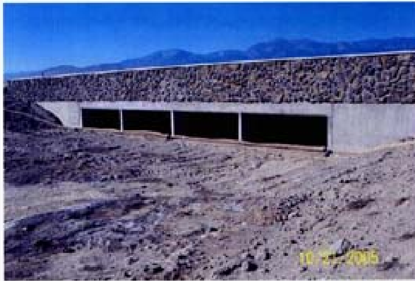
Photo 26. 10/21/05 - Culverts draining channel shown in previous photo. Filter rolls installed at entrance to culverts, apparently intended to provide sediment control.
