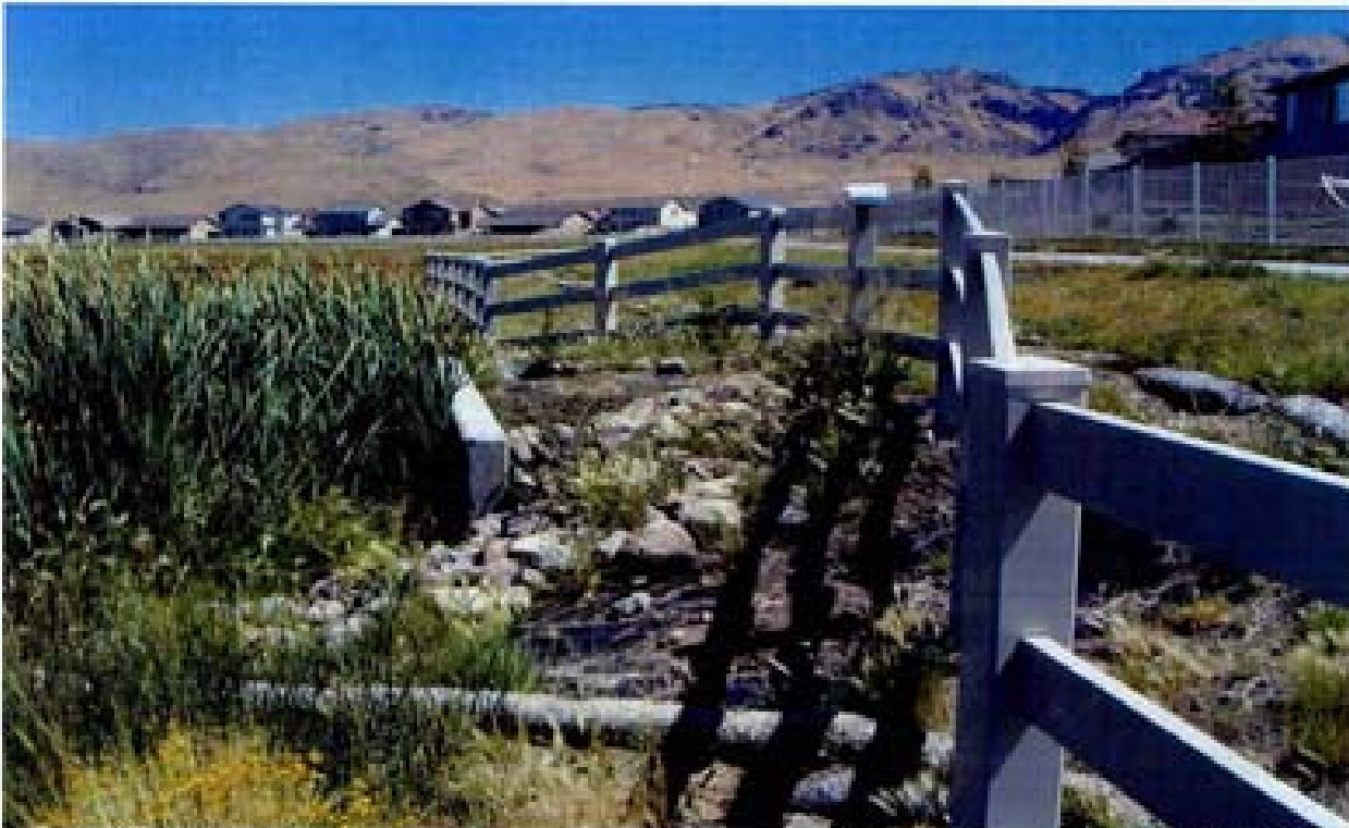
Title: Site 13 - SD out of Village 16 File: HPIM2273.JPG Date: 8/22/2006 12:45 Desc: Slide: 2271 Facing Easterly, outlet of SD and headwall. Heavy growth at culvert outlet. Riprap around headwall is intermittent and geotextile is exposed. Some degradation to corner and side of headwall is visible.
