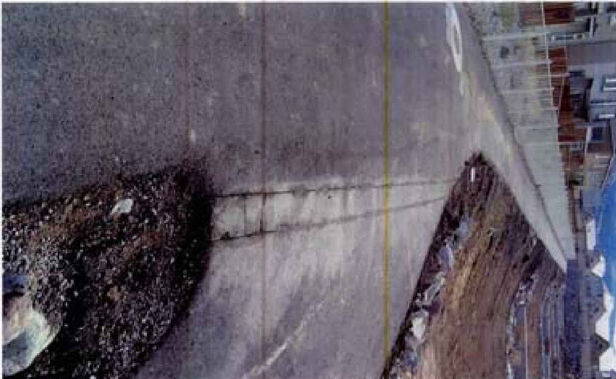
Title: Site 11 SE-8A Channel File: HPM2604.JPG Date: 11/12/2008 11:14 Desc: Slide: 2604 Facing Easterly; top of access road into end of SE-8A channel. Sawcut AC appears to have the cut portions put back into the cut, i.e. inadequate AC patch.
