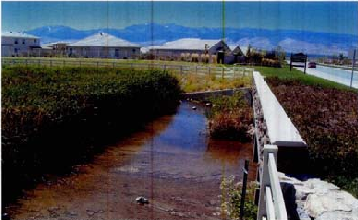
Title: Site 19 - Intersection of Rio Wraspler and Steamboat Parkway File: HPM2296.JPG Date: 8/22/2008 13:53 Desc: Slide: 2293 Facing Westery; upstream apron, wingwall, and headwall of the 5 RCOT's.
