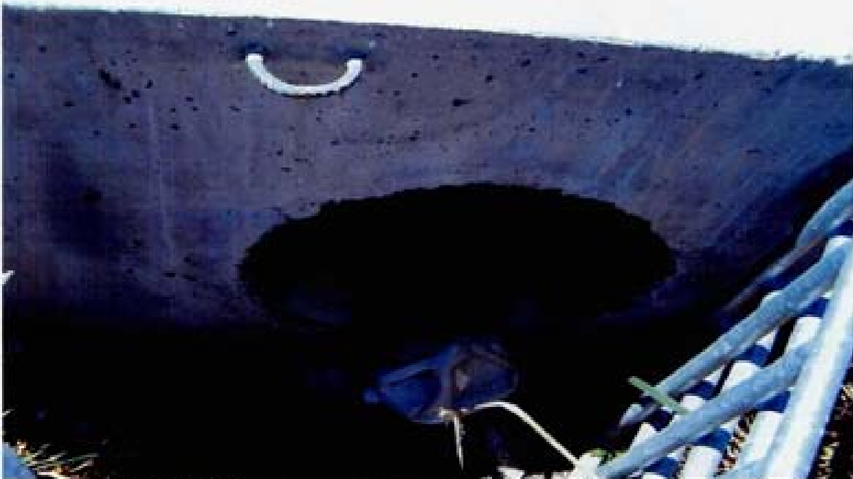
Title Site 16 - SD out of Village 14 File HPIM0282.JPG Date 8/22/2006 13:06 Desc: Facing Westerly; outlet of PVC SD. Headwall/PVC interface is not flush. There are lots of air voids on the face of the headwall. Slide 2280
