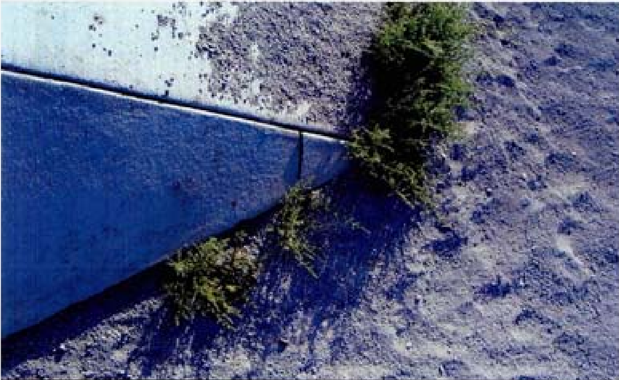
Title: Site 1 - Diversion Structure File: HPIM2238.JPG Date: 8/22/2008 8:53 Desc: Facing NWesterly; top corner of diversion structure at the North end on the detention basin side. Corner of PCC has broken.
