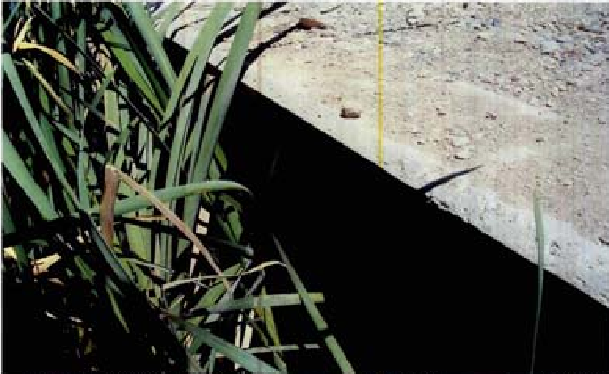
Title: Site 19 - Intersection of Rio Wrangler and Steamboat Parkway File: HPM2291.JPG Date: 6/22/2006 13:47 Desc: Facing East; outlet of RCP. This headwall is poorly formed or was constructed from some sort of pre-cast material.
