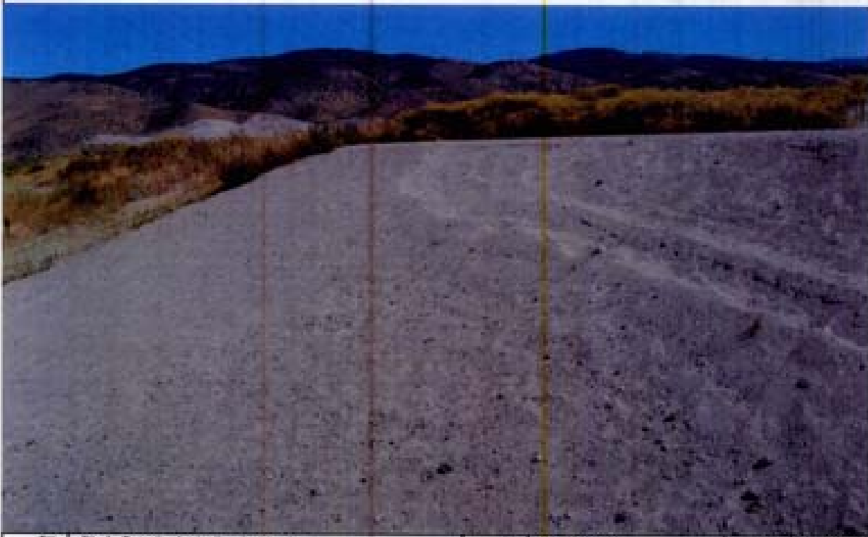
Title: Site 1 - Detention basin diversion structure File: HPM02190.JPG Date: 8/15/2008 15:26 Desc: Facing SEasterly; Soil cement adjacent to diversion structure. Soil cement appears to be sand, non-cohesive down to a depth of about 6 inches.
