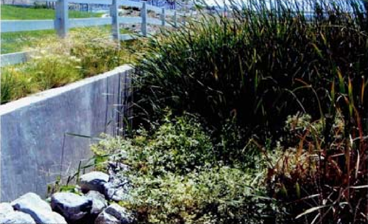
Title: Site 18 - RCB outlet across from Damonite High School File: HPIM0286.JPG Date: 8/22/2008 13:33 Desc: Slide: 2284 Facing SEasterly; outlet of twin RCB's. Heavy vegetation growth at outlet.
