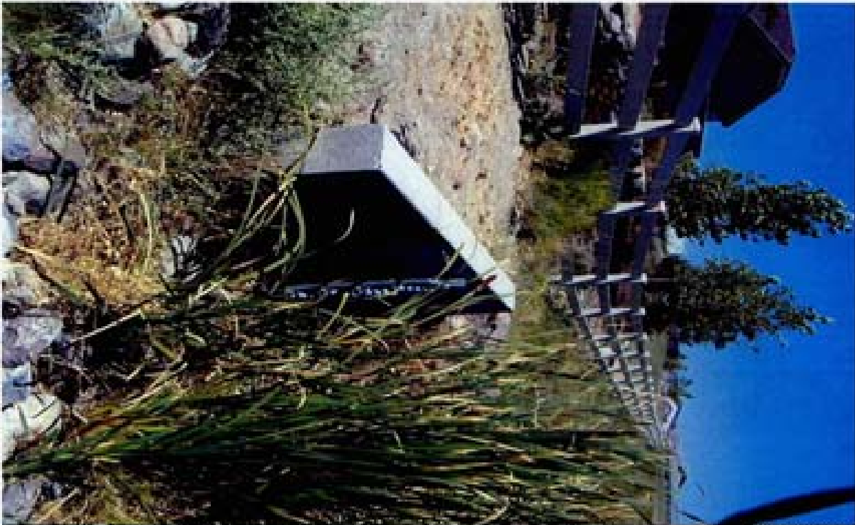
Title Site 16 - SD out of Village 14 File HPIM0281.JPG Date 8/22/2006 13:05 Desc: Facing Northerly; outlet of PVC SD. Headwall and safety grate are visible. Riprap ed protection is visible. The riprap is non-fractured face and uniform in width to length ratio. Slide 2279
