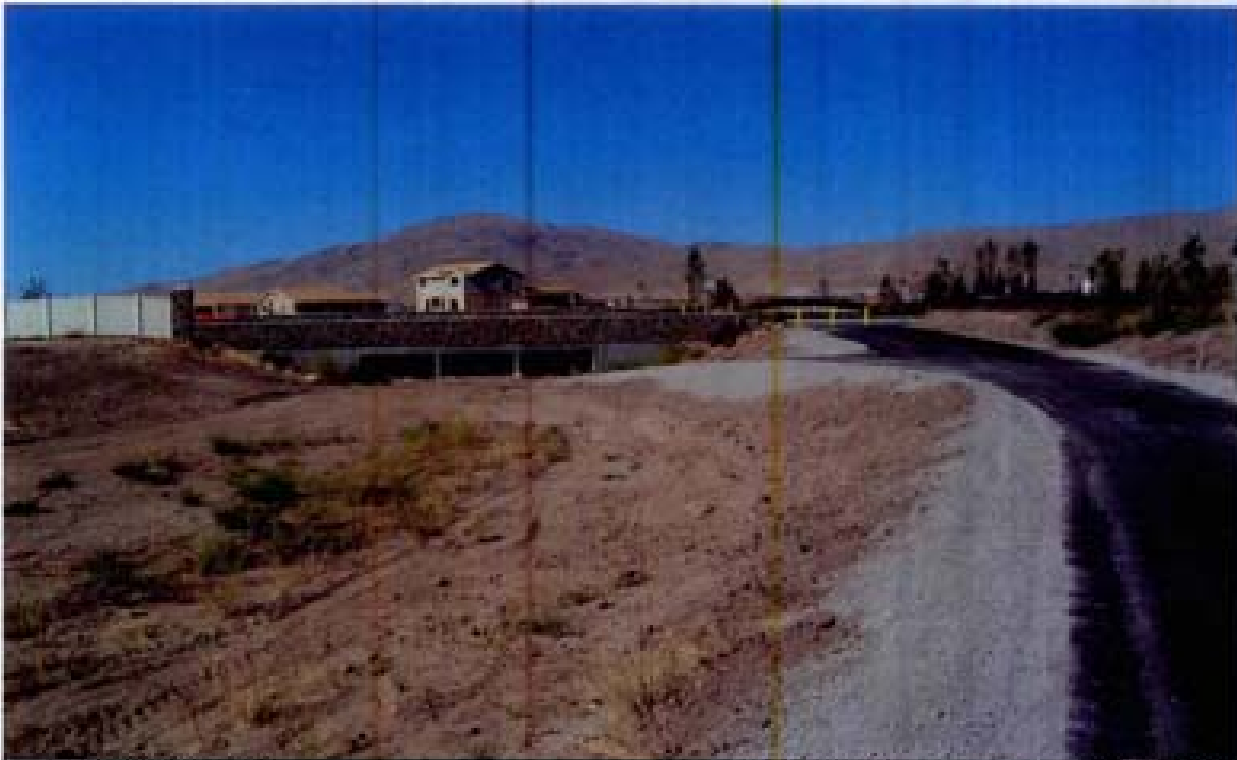
Title: Site 7 - Channel C-5 File: HPM2217.JPG Date: 8/15/2008 16:27 Desc: Facing NEasterly; crossing under rio Wrangler. Earthen channel with little or no vegetation. No grouted riprap protection of access ramp.
