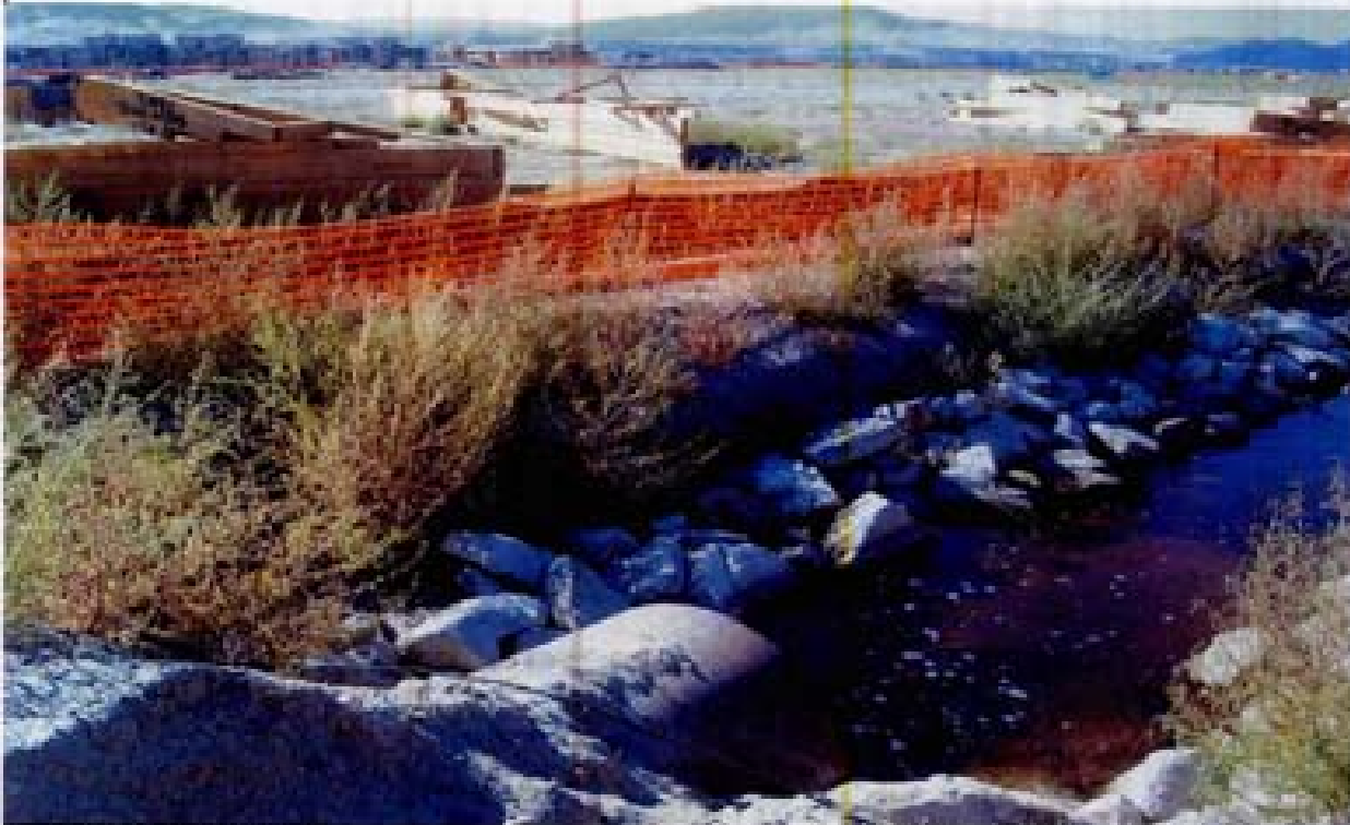
Title: Site 9 - Channel W1-B File: HPM2230.JPG Date: 8/15/2008 16:54 Desc: Slide: 2230 Facing NWesterly, portion of channel directly below the temporary crossing. Poodly constructed riprap channel has collapsed at left bank. There is no underlayment apparent in this portion of collapsed bank.
