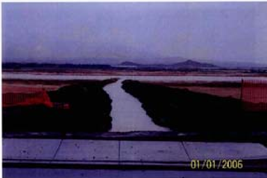
Photo 25. 1/1/06 - View across Rio Wrangler Parkway from previous photo. New drainage ditch discharging to southern section of wetland DE 1. View looking west.
