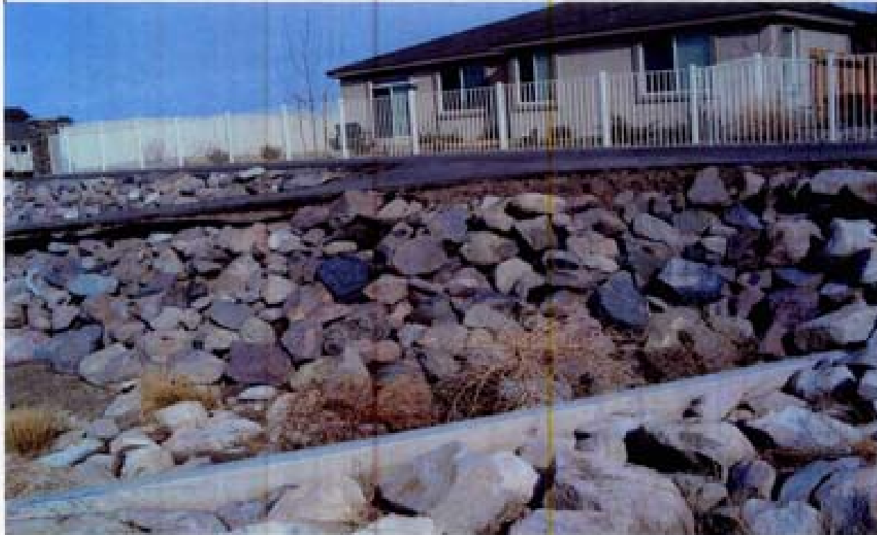
Title: Site 11 SE-8A Channel File: HPM2605.JPG Date: 11/12/2008 11:15 Desc: Slide: 2605 Facing Northwely; riprap on slope of access road is being constructed.
