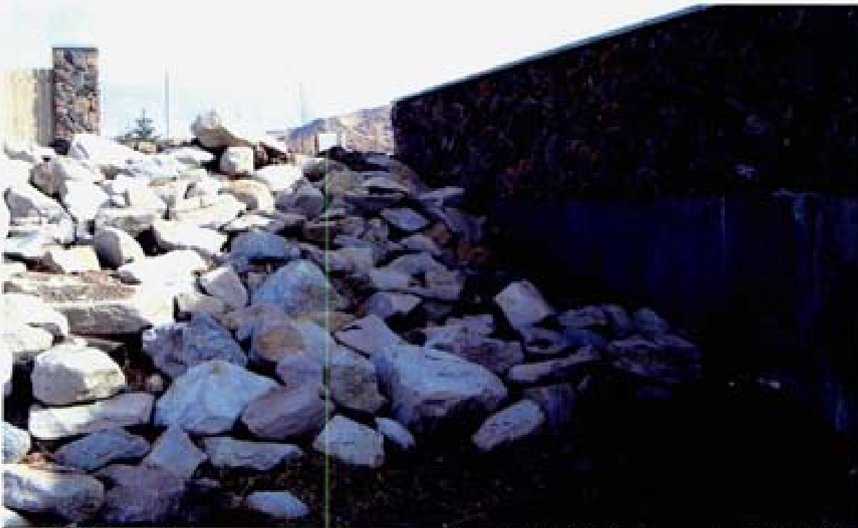
Title: Site 10 W-3 Channel File: HPM2594.JPG Date: 11/12/2008 11:11 Desc: Slide: 2594 Facing Easterly; close up of riprap and wingwall of RCB headwall. The riprap does not appear to have been "toed" into the channel bottom.
