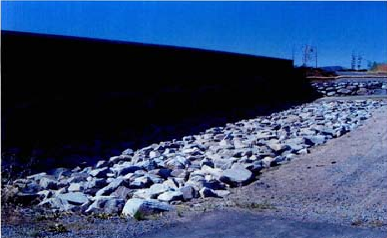
Title Site 3 - Detention basin RCB culvert outlet File HPM2203.JPG Date 8/15/2006 15:54 Desc: Slide 2203 Facing Northerly, outlet of RCB culverts from detention basin. Riprap and outlet appear to be stable. Could not determine depth of riprap or type of underlayment/bedding.
