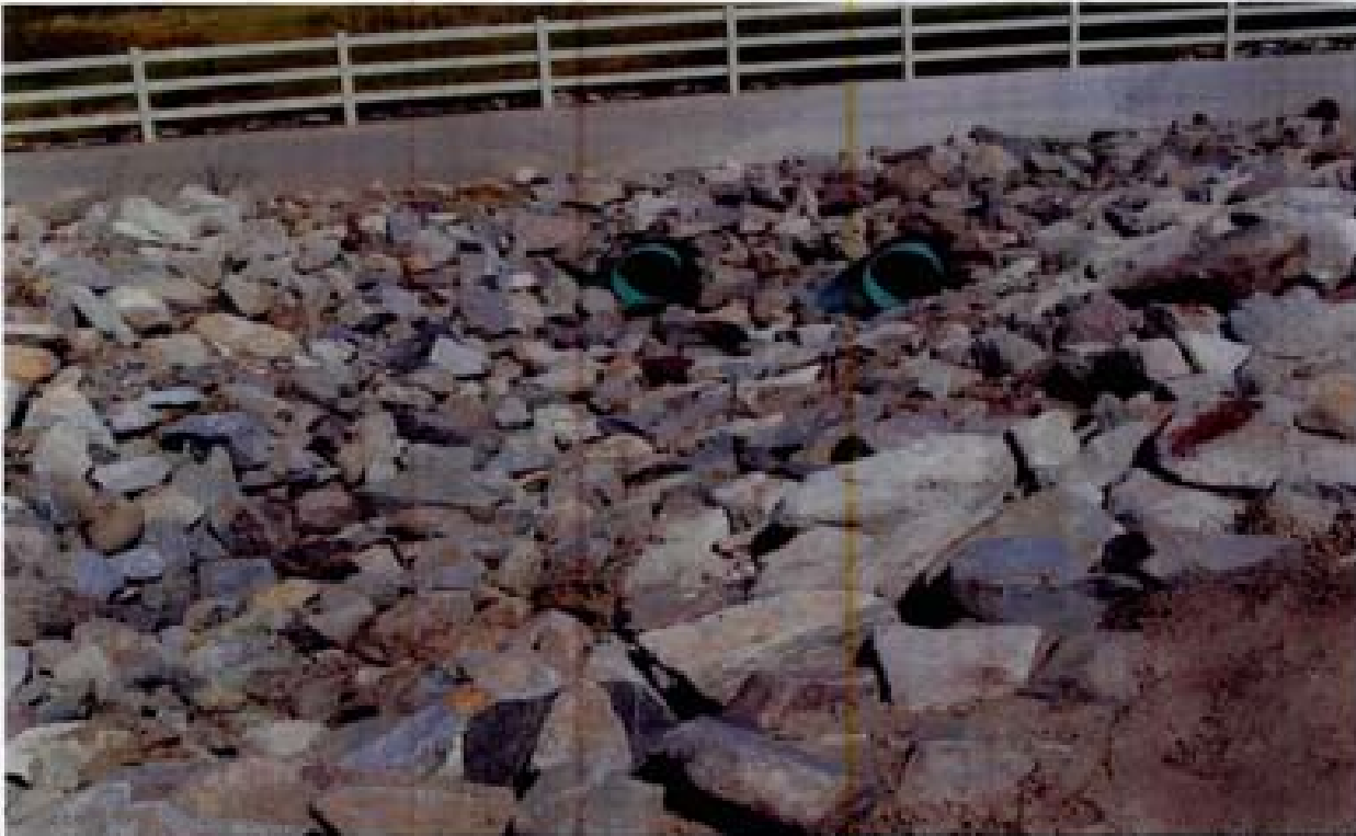
Title: Site B - Channel W1-B File: HPM2271.JPG Date: 8/22/2006 10:56 Desc: Slide: 2269 Facing NEasterly; inlet of low flow PVC pipes with FES. Same location as Photo 2268.
