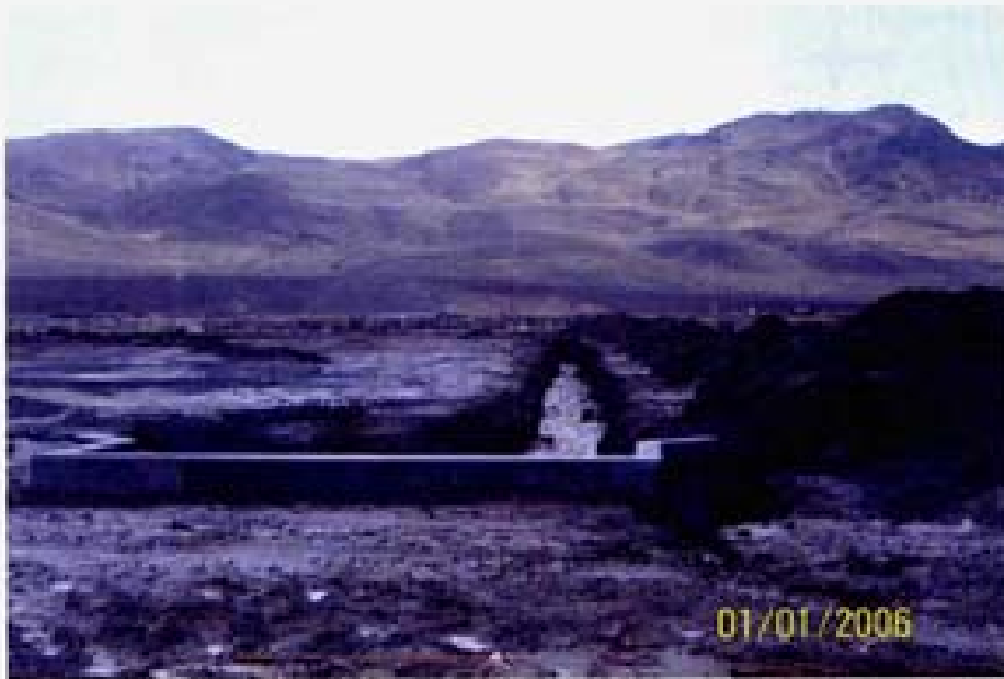
Photo 24. 1/1/06 - New drainage ditch in construction area above Rio Wrangler Parkway draining to southern section of wetland DE 1. No erosion or sediment control BMPs were observed. View looking east.
