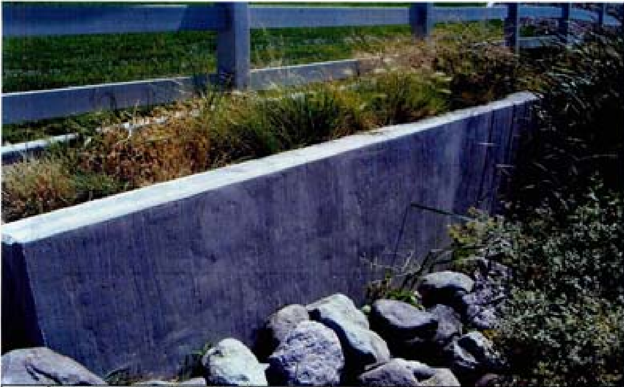
Title: Site 18 - RCB outlet across from Damonite High School File: HPIM0285.JPG Date: 8/22/2008 13:33 Desc: Slide: 2283 Facing SEasterly; wingwall of twin RCB's and RCP SD. Face of headwall/wingwall has been refinished. Riprap is non-fractured face and some are of uniform length/width ratio.
