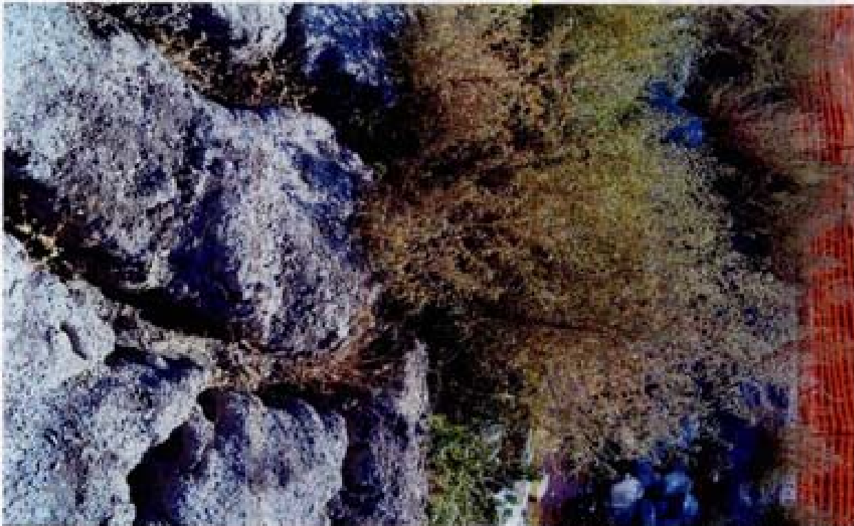
Title: Site 9 - Channel W1-B File: HPM2229.JPG Date: 8/15/2008 16:54 Desc: Slide: 2229 Facing Westery, portion of channel downstream of Rio Wrangler... below temporary crossing. Storm flow from adjacent undeveloped parcel has eroded, contributing sediment to the channel and undermined the riprap.
