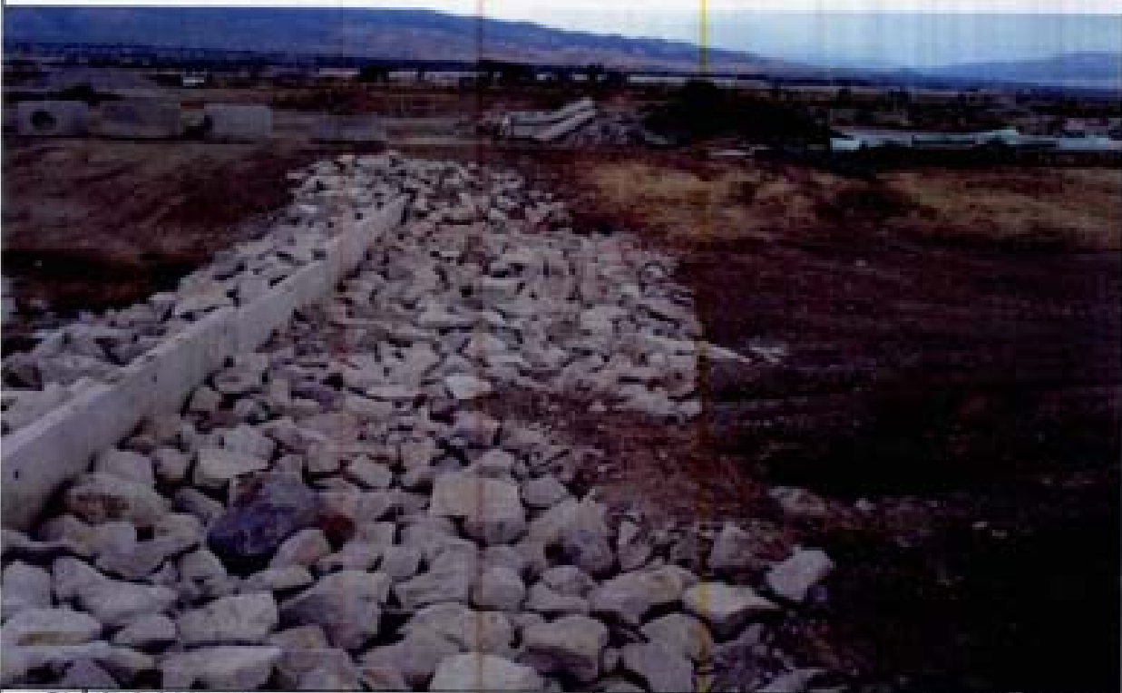
Title: Site 7 - C-5 Channel File: P1010158.JPG Date: 9/18/2006 15:17 Desc: Facing Westerly; second grade control sill downstream of RCB outlet. The grade upstream of the sill appears to be the same as downstream of the sill. This is consistent with what is observed at the first grade control sill in Photo 1010150. There are no visible signs of riprap underlayment.
