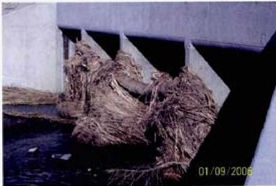
Photo 8, 10/06 - Close-up of debris trapped between culverts after 10/05 storm event.
