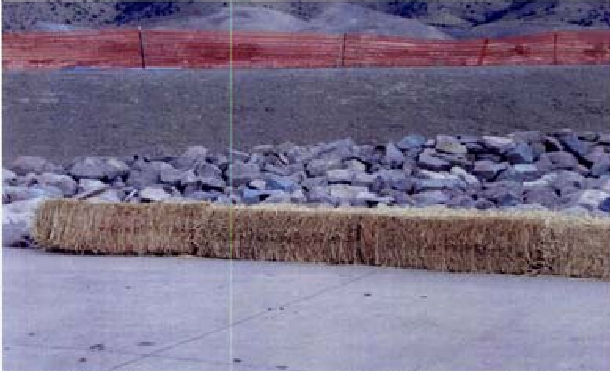
Title: Site 6 - Channel C-7 File: P1010176.JPG Date: 9/18/2006 15:17 Desc: Slide: 1010176 Facing Easterly; straw bales placed for sediment control at end of C-7 channel. These hay bales are not embedded into the sub-grade and do not appear to be staked in.
