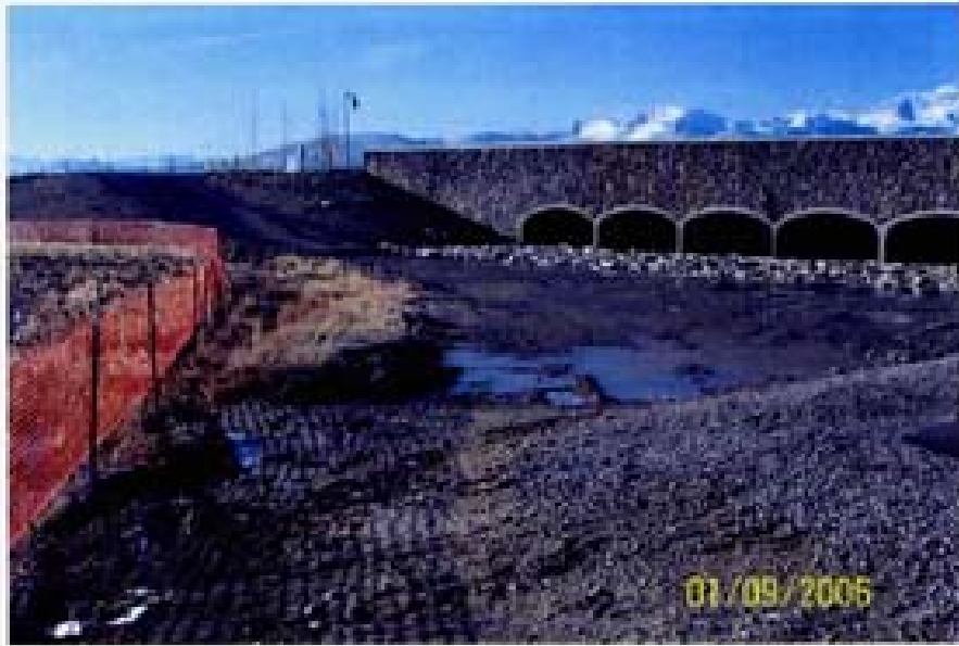
Photo 16. 1556 - Culverts under Pioneer Parkway. View looking southeast of culvert outlets just above west end of wetland D65 after 12/31/05 storm event.
