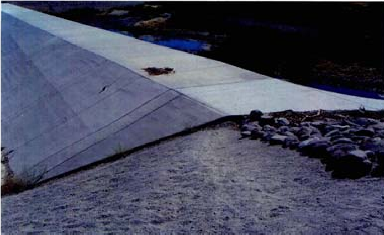
Title: Site 1 - Detention basin diversion structure File: HPIM2199.JPG Date: 8/15/2006 15:38 Desc: Facing Southerly; at North end of diversion structure. Note same non-cohesive sand layer. Riprap at end of structure is single layer of rock with no bedding or geotextile.
