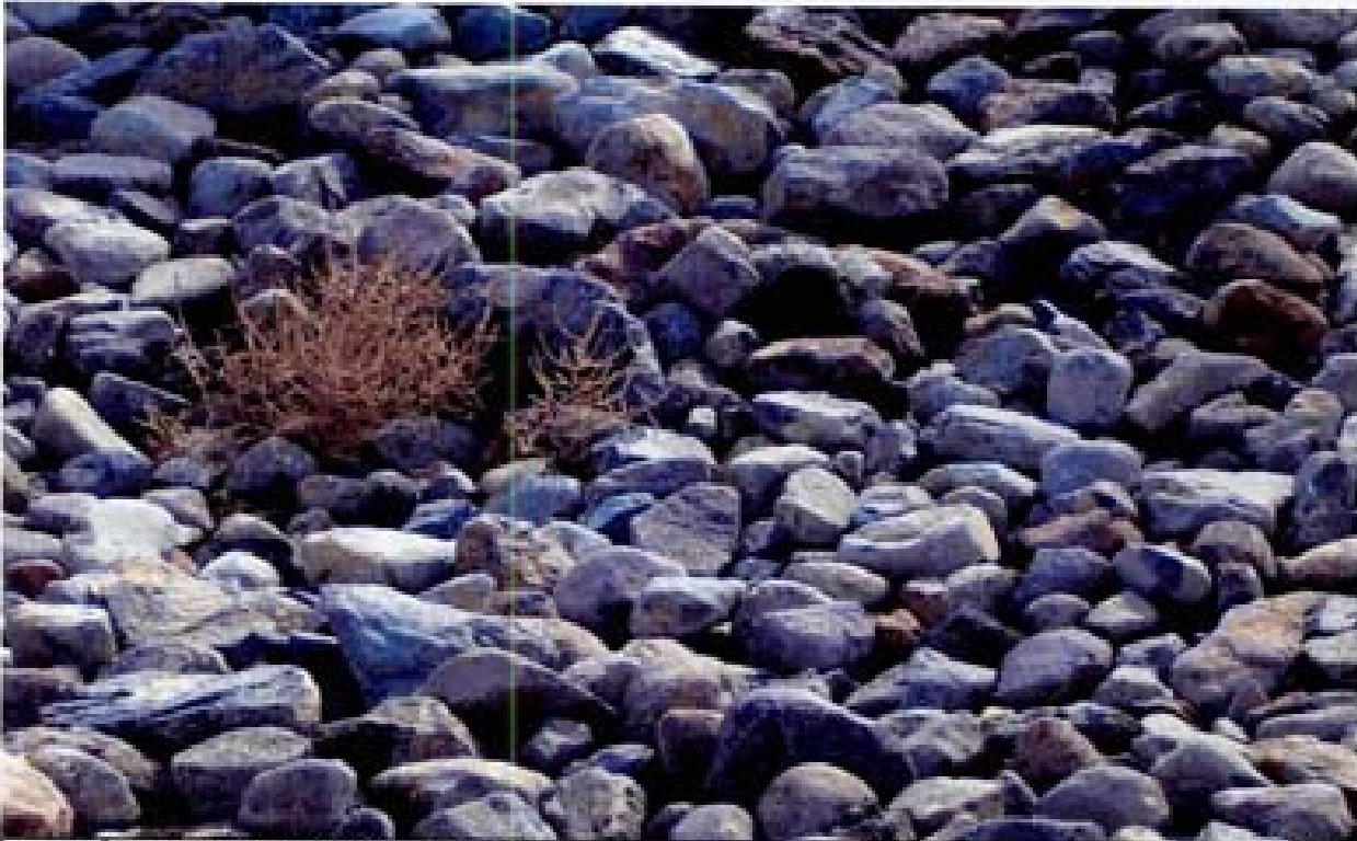
Title Site 18 Damonte High School Boundary Channel File HP1M0810.JPG Date 11/12/2006 11:21 Desc Slide 2610 Facing southerly; close up of riprap used to line the damonte High School Boundary Channel. Riprap appears to be a very small rock with poor gradation; i.e. large amounts of small rock.
