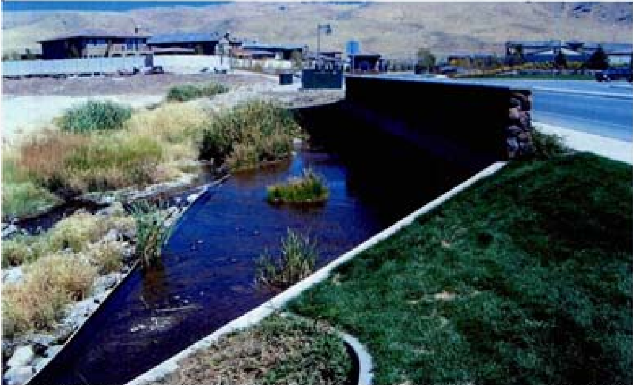
Title: Site 19 - Intersection of Rio Wrangler and Steamboat Parkway File: HPIM2295.JPG Date: 8/22/2006 13:51 Desc: Slide: 2292 Facing Easterly, downstream outlet of RCB's. The riprap apron at the end of the PCC wingwall apron appears to be highly disturbed or poorly constructed. The vegetation in the left background is masking an earthen berm that forms a channel that the RCP SD pictured in photo 2290 discharges into.
