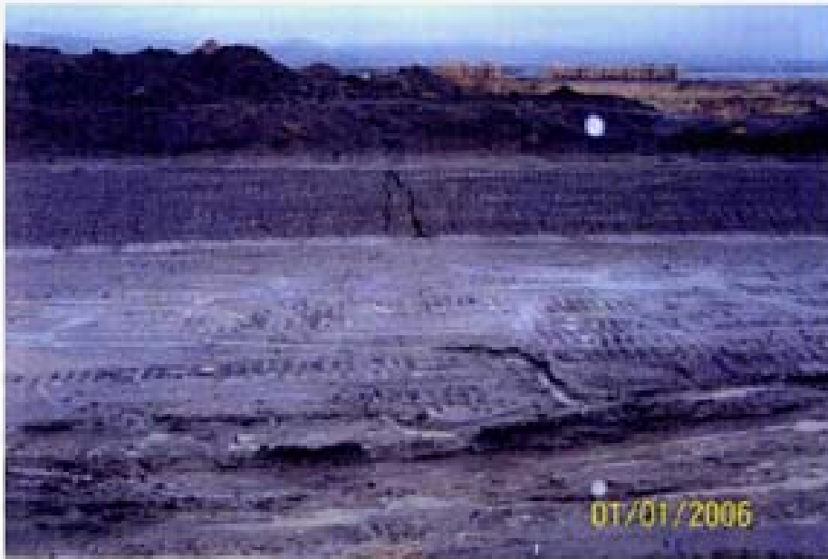
Photo 58. 1/1/06 - Erosion in channel W-1. Note that dune tracks parallel with slopes accelerated erosion.
