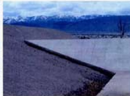
PCC weir and soil cement interface. Erosion and undercutting of weir.
