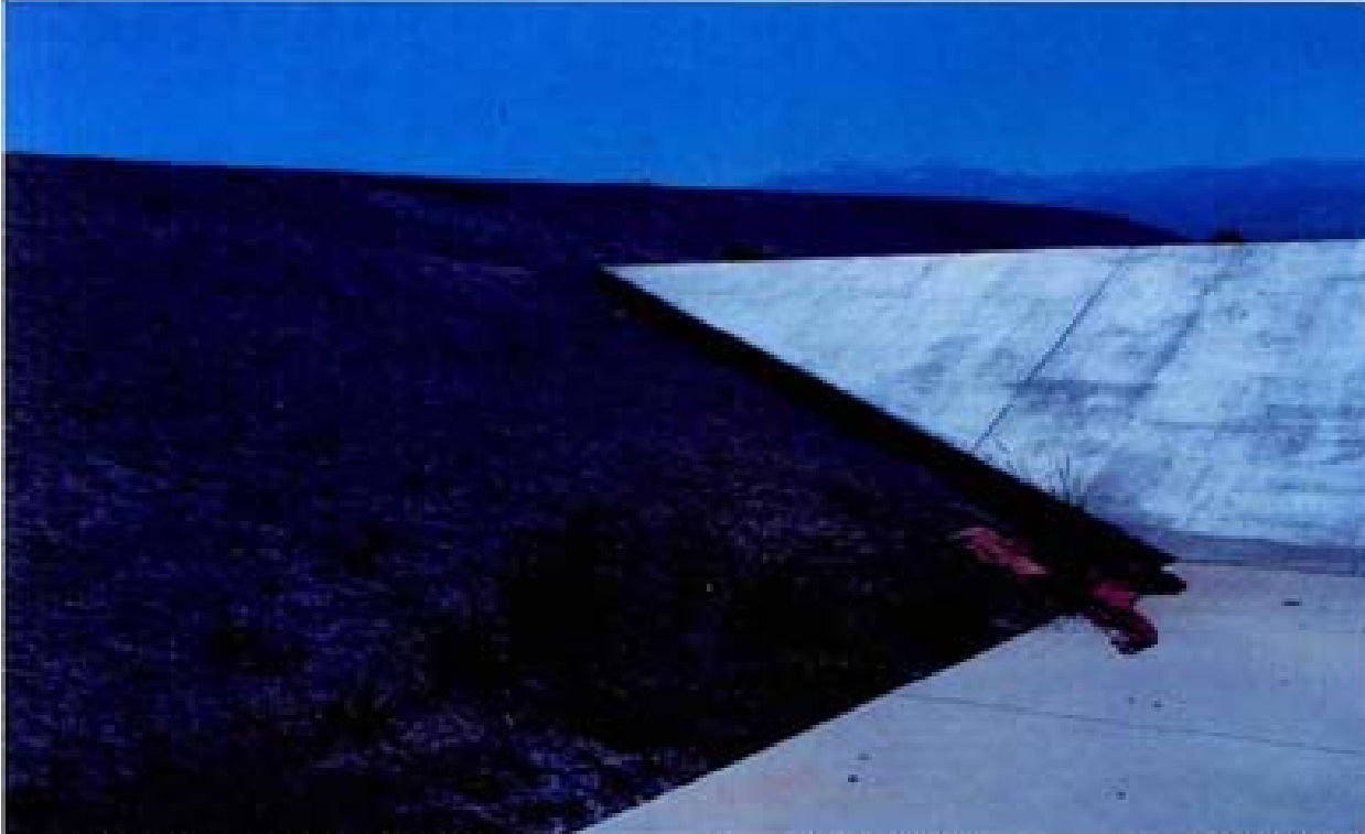
Title: Site 1 - Detention basin diversion structure File: HP0M2192.JPG Date: 8/15/2006 15:27 Desc: Facing Westerly; South corner of diversion structure. Sand/soil cement has eroded away from end of PCC diversion structure. No cutoff wall constructed at ends of PCC diversion structure.
