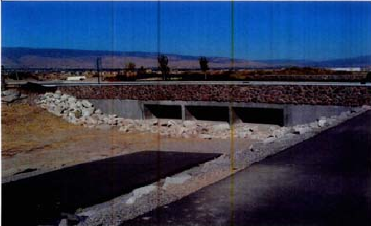
Title: Site 11 - Channel SE-4A File: HPM0247.JPG Date: 8/22/2006 10:03 Desc: Slide: 2246 Facing NEasterly; channel C-5 and inlet to RCB's under Rio Wrangler. Riprap stabilization of box culvert inlets. Access ramp in foreground of photo. Riprap protection of side slopes.
