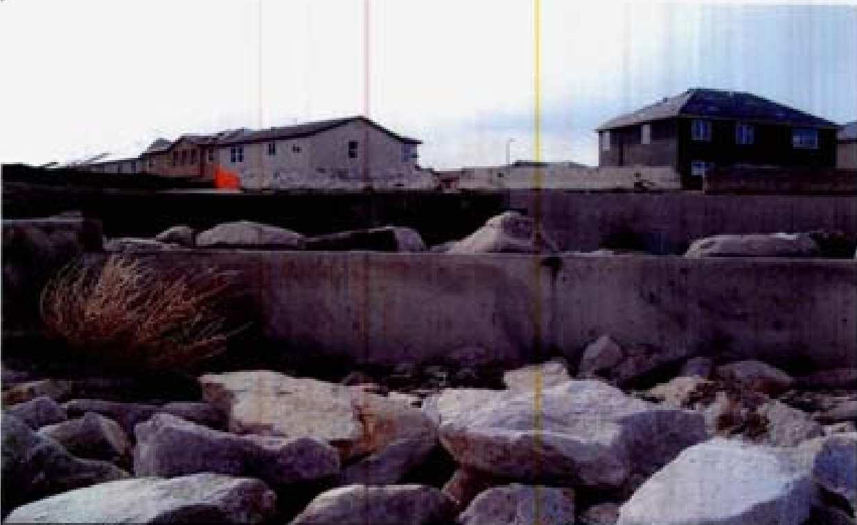
Title: Site 7 Channel C-5 File: HPMG585.JPG Date: 11/12/2008 11:01 Desc: Slide: 2585 Facing South; same as above slide 2584 panning right. Honeycombing and sebacks not filled in. This photo taken ~ level; note the difference in grade between the top of the grade control sill and RCB invert in background.
