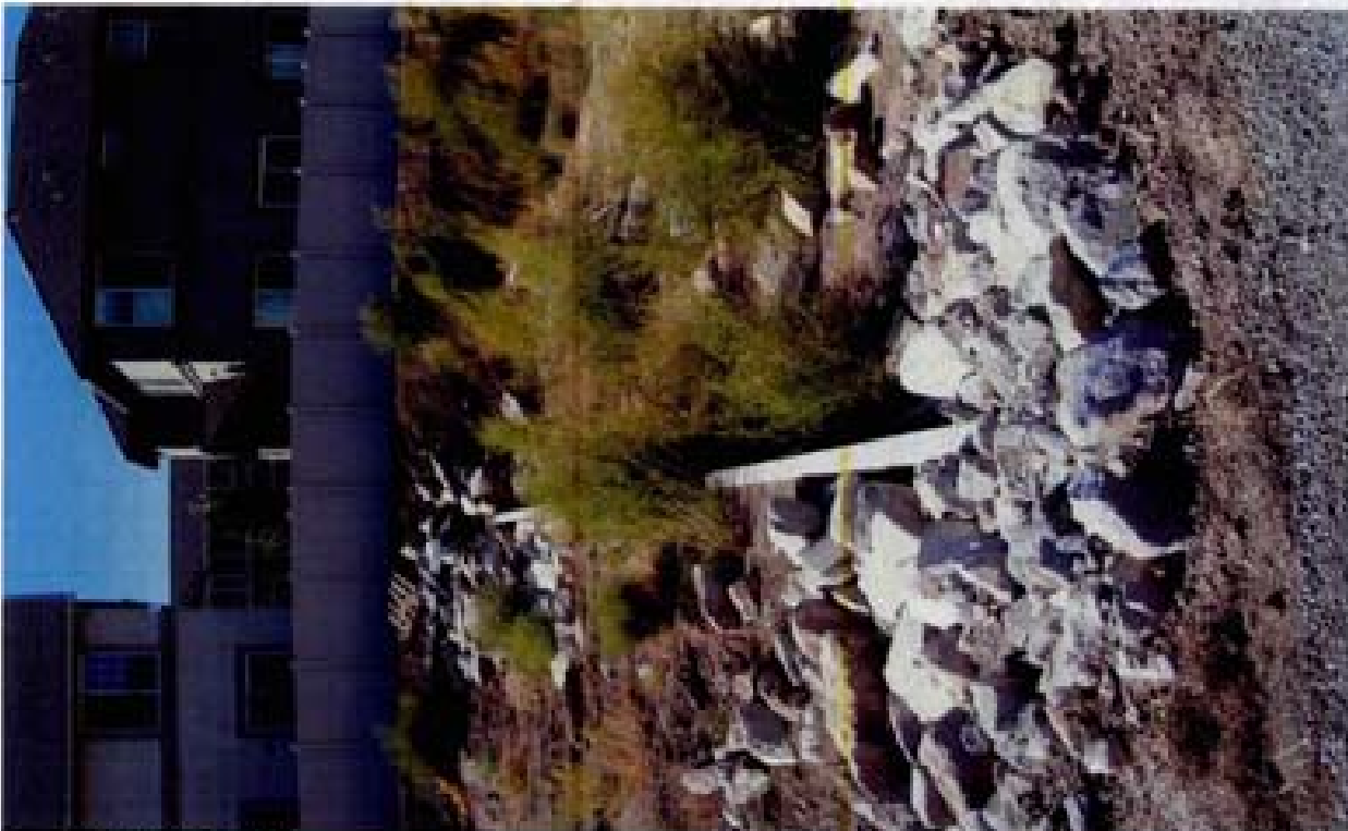
Title: Site 7 - Channel C-5 File: HPM2221.JPG Date: 8/15/2006 14:35 Desc: Slide: 2221 Facing NWesterly; grade control sill up gradient of Rio Wangler. Poorly placed riprap with no apparent underlayment or bedding. The riprap in the background has been placed after the silt fence was installed and appears to have just been dumped as opposed to placed. Typical situation in this channel was the pushing of adjacent construction material into the channel. Silt fence has been crushed by riprap.
