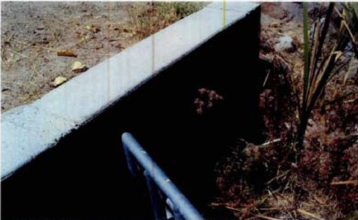
Title Site 16 - SD out of Village 14 File HPM2283.JPG Date 8/22/2006 13:06 Desc: Slide 2281 Facing Westerly. Outer face of headwall. More air voids in face of headwall. Note the poor finishing of the PCC along the top of the headwall.
