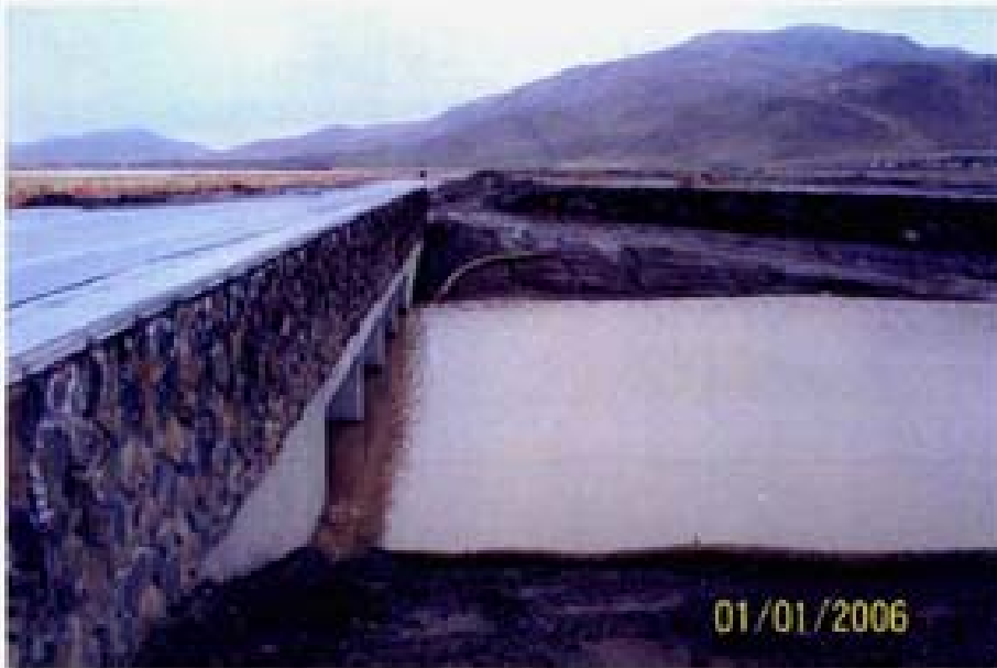
Photo 30. 1/1/06 - Same view as previous photo after 12/31/05 storm event.
