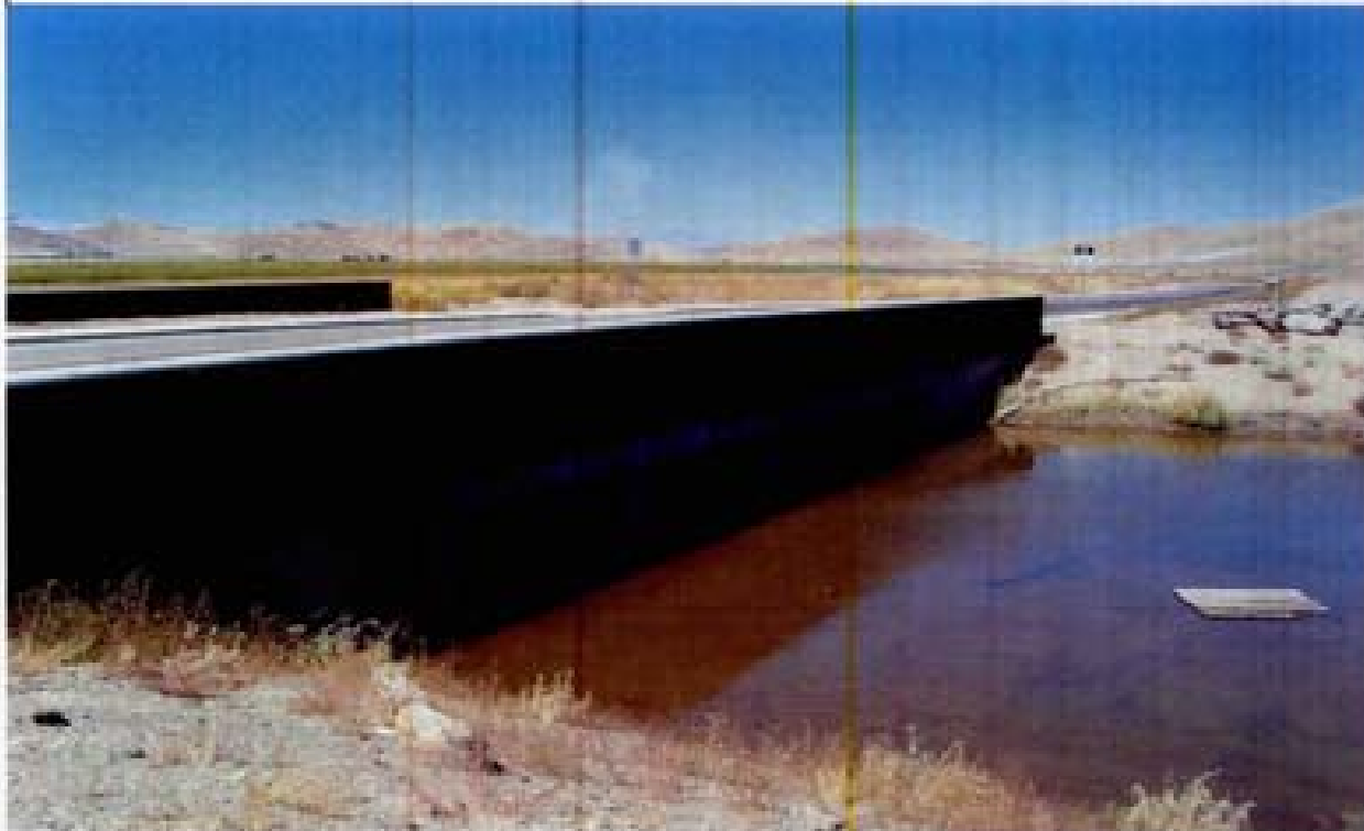
Title: Site 20 - bridge crossing under Rio Wraspler South of Steamboat Parkway File: HPM2297.JPG Date: 8/22/2008 13:59 Desc: Slide: 2294 Facing NWestery; upstream inlet of 4 RCOT's. Channel is eaten with water ~0.5 feet deep.
