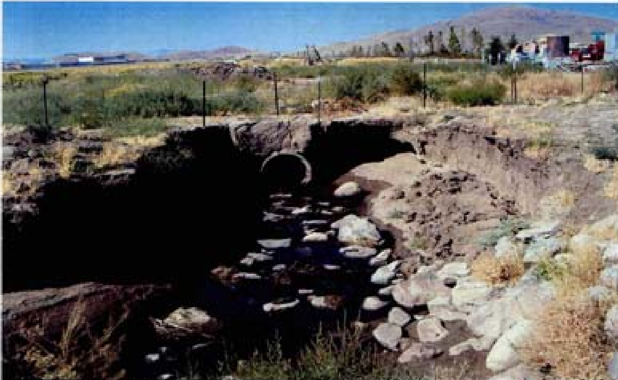
Title Site 5 - Crane & Clow Ditch File HP1M2215.JPG Date 8/15/2006 16:16 Desc: Facing Northerly; portion of rerouted ditch after the 90 degree turn shown in the background of Photo 2214. This portion also show signs of being very unstable and the developer has attempted to stabilize in the past with a layer of riprap visible in the right foreground. The sidewalls are near vertical and have collapsed from a probable combination of undercutting and pore pressure. The culvert appears to be undersized, lacks a headwall and has eroded significantly.
