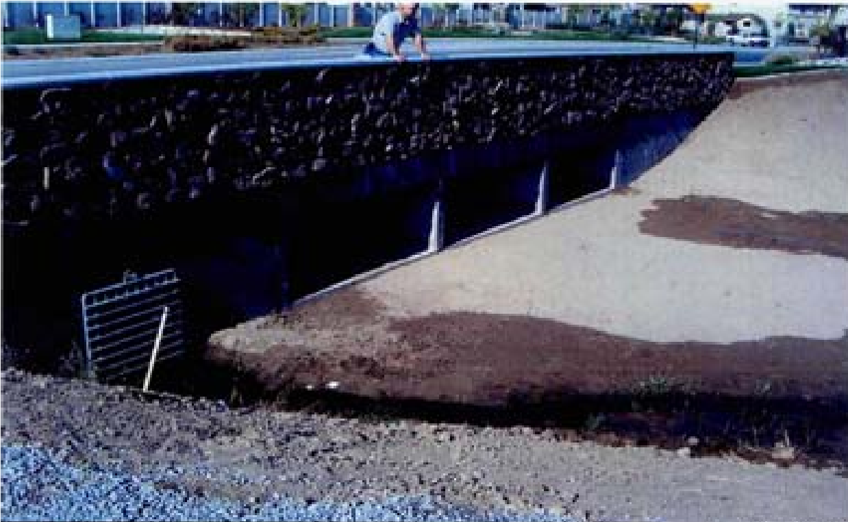
Title Site 7 - Channel C-7 File HPIM2244.JPG Date 8/22/2008 9:44 Desc: Facing Westerly; downstream outlet of RCB's under Rio Wrangler. Safety grate on SD outlet no longer applicable per Reno Standard Details. Channel is earthen with no vegetation. No riprap stabilization of accessramp in bottom foreground of photo.
