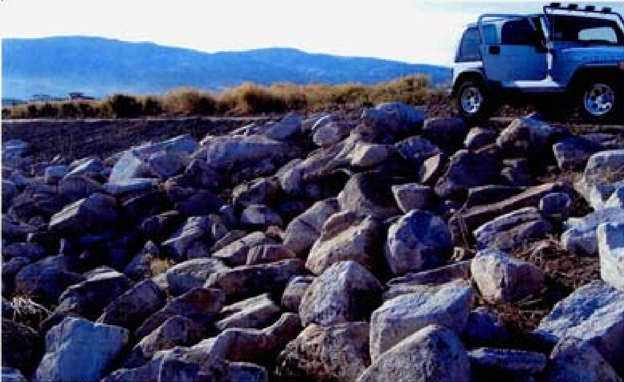
Title Site 2 - Detention Basin File HPIM2232.JPG Date 8/22/2006 8:27 Desc: Slide 2232 Facing SEasterly, same location as Photo 2231. Developer has backfilled and ripraped the erosion gully that was documented on 08/15/06 site walk (see description for Photo 2231).
