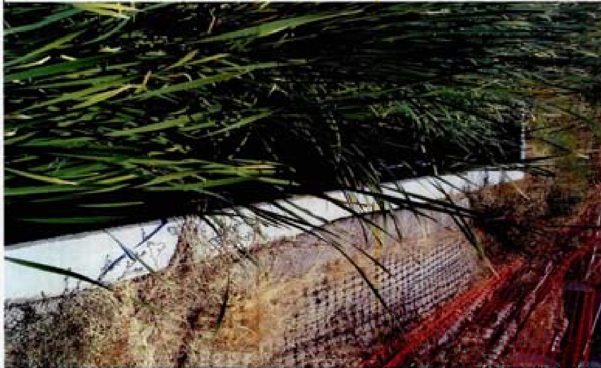
Title Site 14 - SD out of Village 15 File HP1M0276.JPG Date 8/22/2006 12:52 Desc Facing Westerly; headwall at outlet of SD. Heavy vegetation and safety gate are visible.
