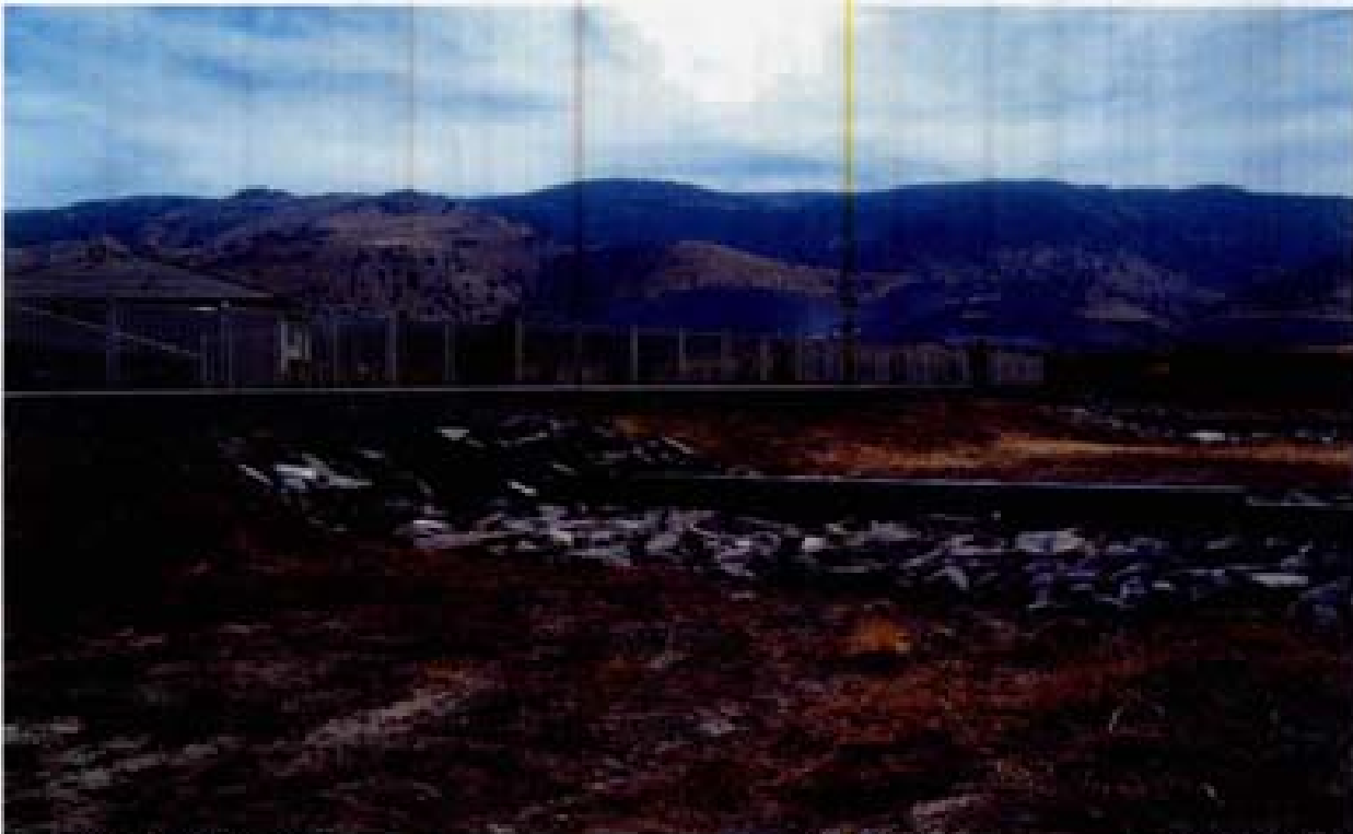
Title: Site 11 - Channel SE-8A File: HPM2254.JPG Date: 8/22/2008 10:12 Desc: Facing Easterly; poorly constructed riprap and protection of control sill. No sign of riprap underlayment or bedding.
