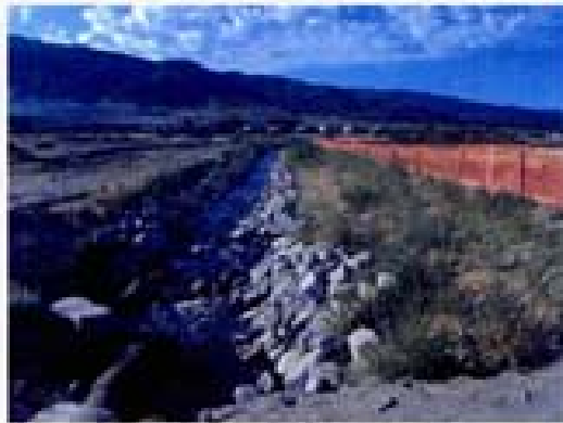
Drainage Channel directing water into the wetlands.
