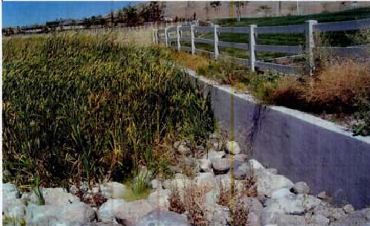
Title: Site 18 - RCB outlet across from Damonte High School File: HPM2288.JPG Date: 8/22/2008 13:36 Desc: Slide: 2286 Facing Northerly; south side of the headwall/wingwall. The RCP is visible in the center of the photo.
