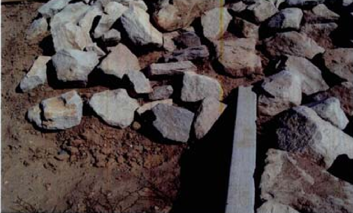
Title: Site 7 - Channel C-5 File: HPM2218.JPG Date: 8/15/2008 16:29 Desc: Facing Easterly; close up of end protection on PCC grade control sill. Riprap is placed poorly with inadequate thickness and no bedding or underlayment.
