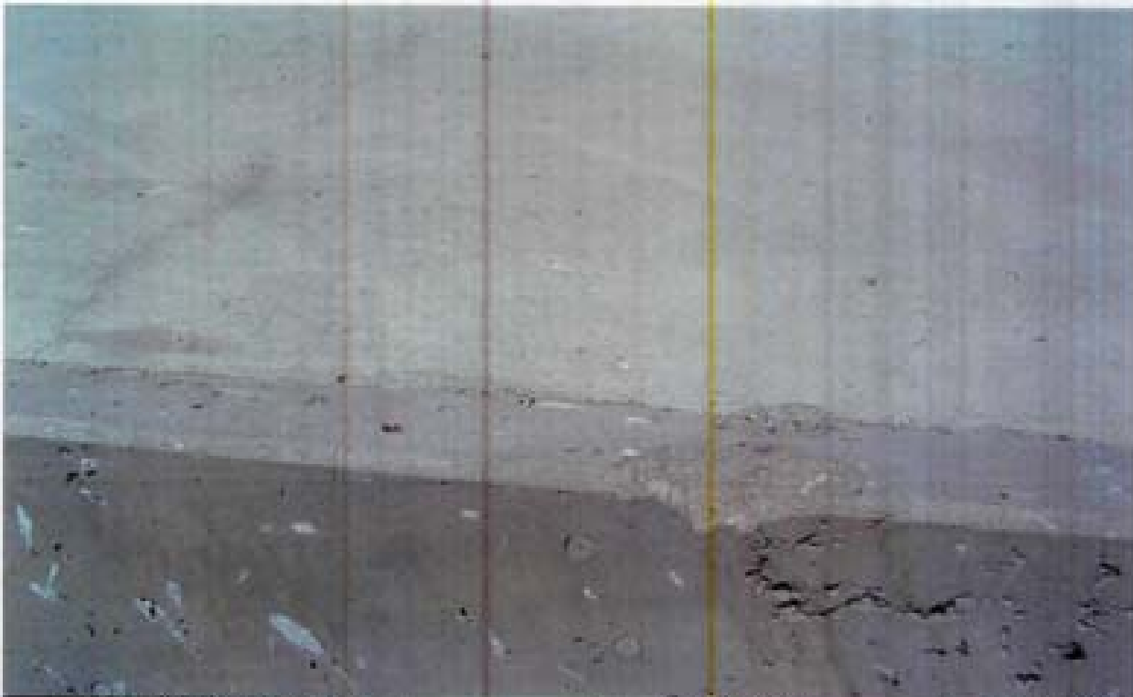
Title Site 1 - Detention basin diversion structure File HPM2197.JPG Date 8/15/2008 15:36 Desc: Facing Easterly, same location as Photo 2196. Note spalled PCC on wing wall and air void from improper vibration of concrete during pour.
