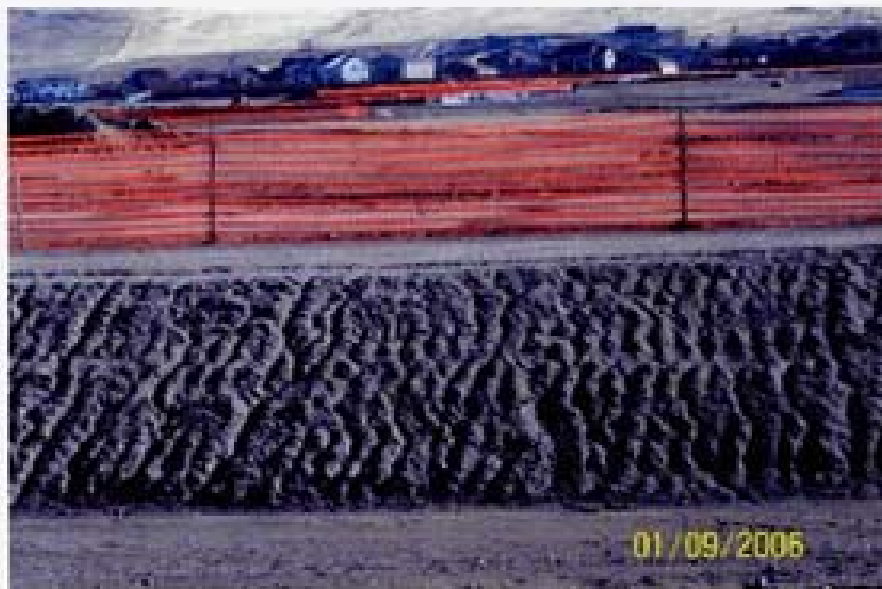
Photo 09, 1/9/06 - Erosion rills in the side slopes of channel C-7 were accelerated because tracking was conducted perpendicular to slope, leaving grooves parallel to slope.
