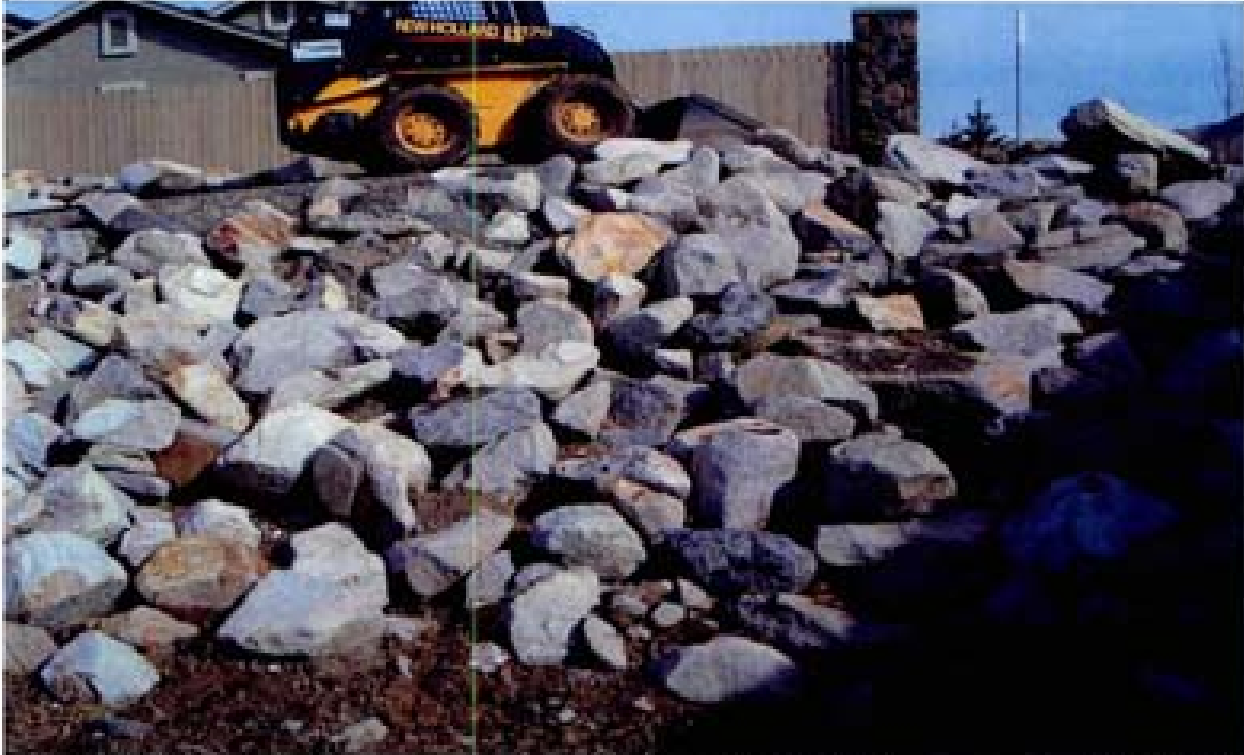
Title: Site 10 W-3 Channel File: HPM2595.JPG Date: 11/12/2008 11:11 Desc: Slide: 2595 Facing Easterly; riprap appears to be of good quality with angular faces and good length to width characteristics. Hard to verify riprap layer thickness.
