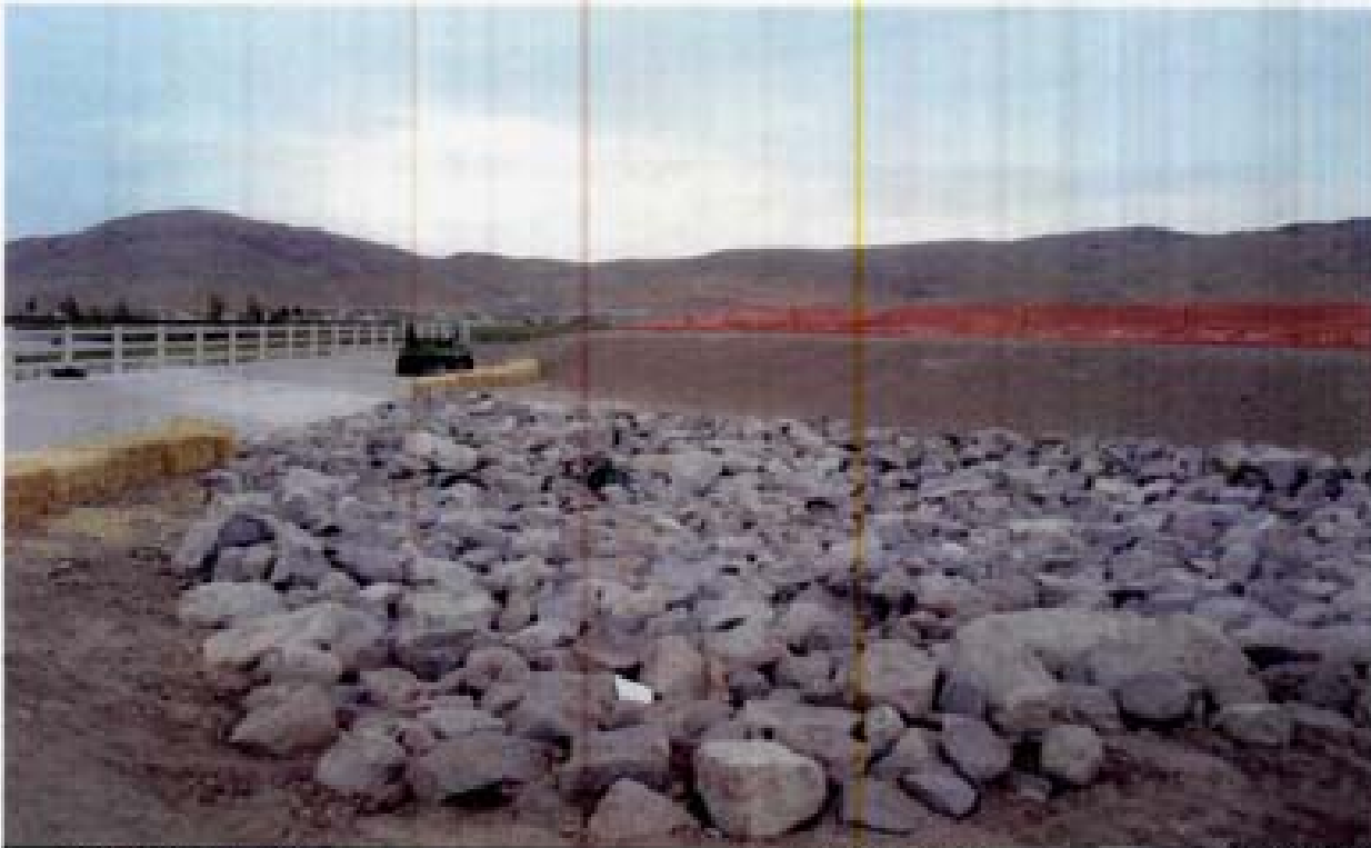
Title: Site 8 - Channel C-7 File: P1010173.JPG Date: 9/15/2006 15:17 Desc: Slide: 1010173 Facing Easterly, outlet of C-7 channel. No sign of underlayment or riprap bedding is visible. The riprap is not excavated into the channel and is not symmetrical with the trapezoidal cross-section of the channel.
