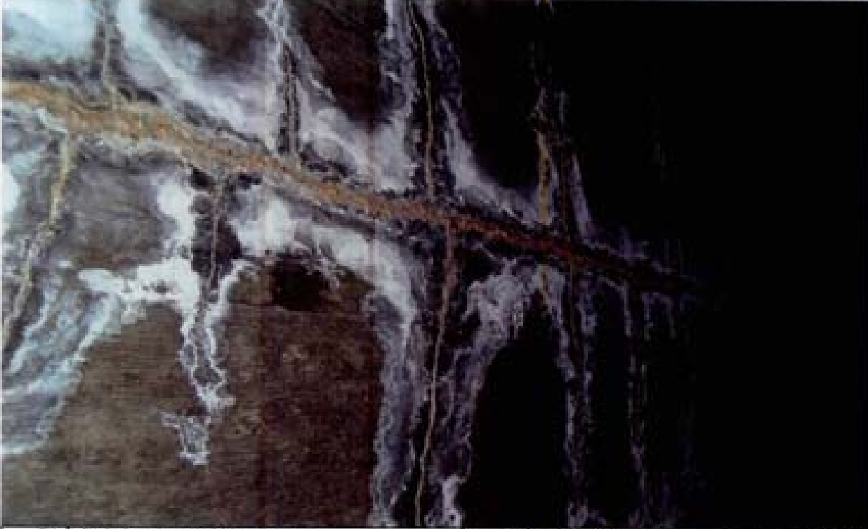
Title: Site 3 - Detention basin RCB culvert outlet File: HPM2202.JPG Date: 8/15/2006 15:52 Desc: Inside the footpath located in RCB at North end of outlet structure. These cracks appear in every panel of the cast in place RCB culverts.
