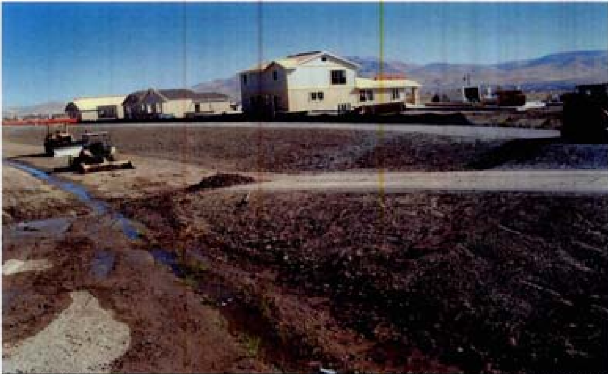
Title: Site 7 - Channel C-7 File: HPM0246.JPG Date: 8/22/2006 9:48 Desc: Slide: 2245 Facing Northerly; construction in channel C-7 downstream of Rio Vista.
