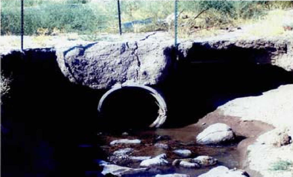
Title Site 5 - Crane & Clow Ditch File HP1M2216.JPG Date 8/15/2006 16:16 Desc: Facing Northerly; same location as Photo 2215. Close up showing erosion from eddies created by lack of headwall and high entrance velocities to culvert.
