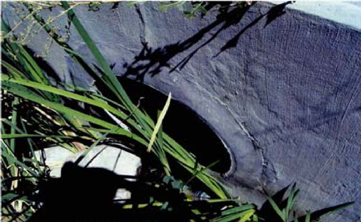
Title: Site 18 - RCB outlet across from Damonite High School File: HPM02289.JPG Date: 8/22/2008 13:37 Desc: Slide: 2287 Facing NEasterly; Outlet of sd. The face has been refinished at the SD/headwall interface.
