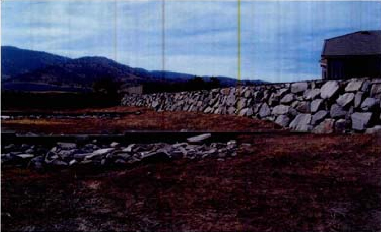
Title: Site 11 - Channel SE-8A File: HPM2255.JPG Date: 8/22/2008 10:13 Desc: Facing SEasterly; grade control sills. No riprap protection of end of control sills. Rockery wall encroaches into flood channel.
