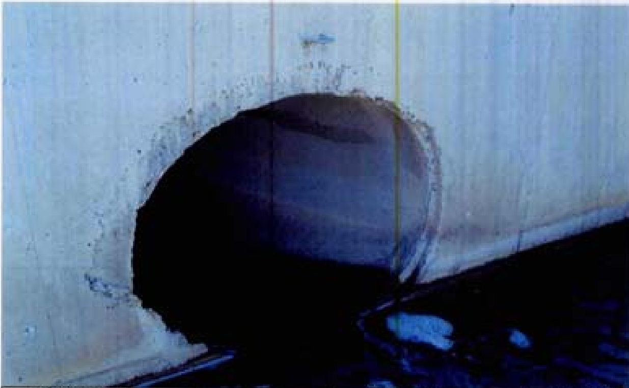
Title Site 4 - DES Wetland File HPM2205.JPG Date 8/15/2008 16:00 Desc: Facing NEasterly; outlet of Crane & Clog into DES wetland. Convent headwall is poorly formed and had flaked away from headwall/RCP interface. End of RCP should be mitered and flush with face of headwall.
