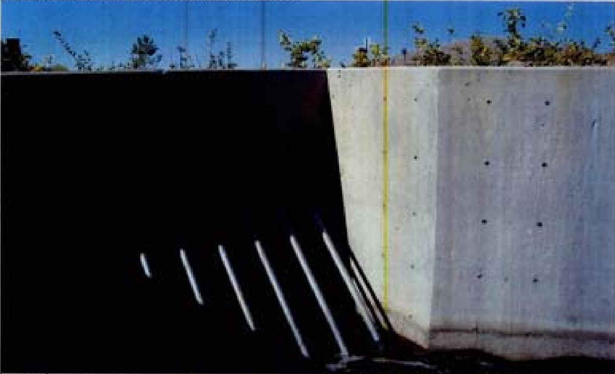
Title: Site 9 - Channel C5-B File: HPM2222.JPG Date: 8/15/2006 16:42 Desc: Slide: 2222 Facing Northerly; Culvert headwall/wing wall for pair of 36 inch RCP's. Form plugs have not been removed and filled.
