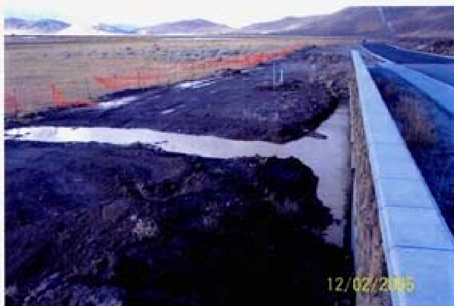
Photo 31. 12/02/05 - Temporary (?) channel installed below culverts shown in previous photo. Culvert invert elevations appear to be below adjacent wetlands and are unable to drain completely. View looking north.
