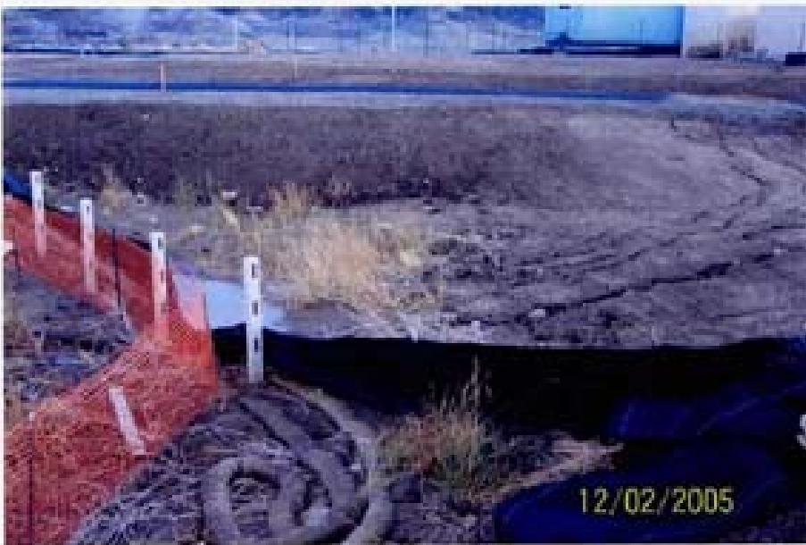
Photo 84. Silt fence near culvert outlet from Crane & Claw ditch needs maintenance.
