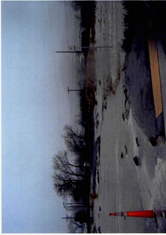
Figure G.15. Bailey Canyon Creek overtopping Toll Road (looking south)
