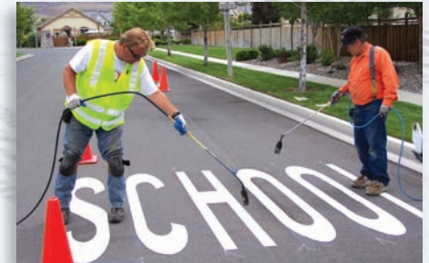
City of Sparks Traffic Maintenance Workers Marty Redding (left) and Dick Kirtley install new heat tape in a school zone.
