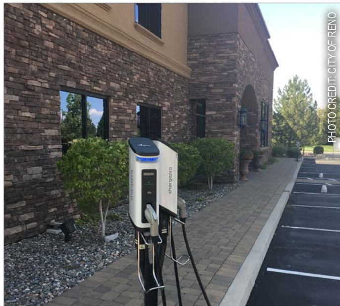
Example: Electric vehicle charging stations
